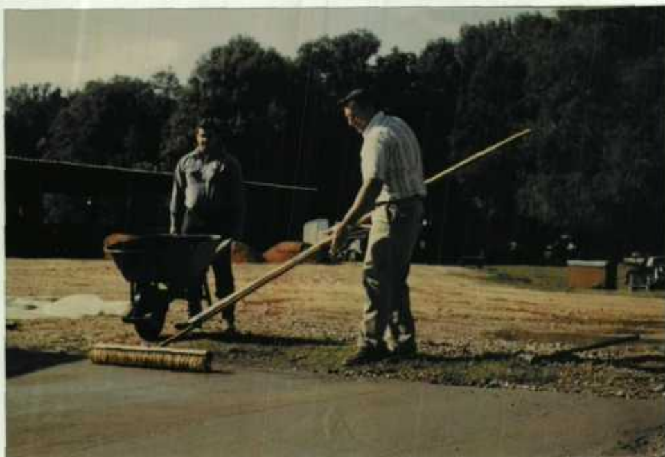
Bill's sunny disposition reflects the weather as the concrete is poured. 11/83 JTF
