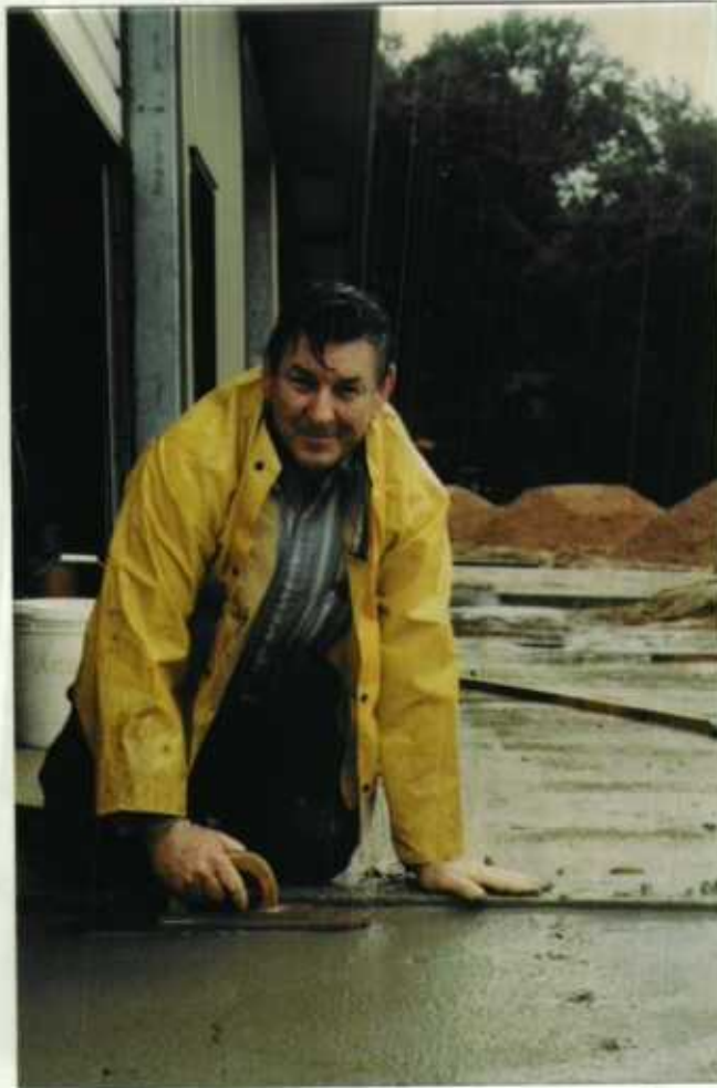
Not even a monsoon can dampen Bill's spirits or distract him as he works the concrete surface to perfection.
