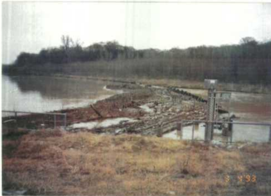
The heavy weight of drift has damaged the drift barrier on the north end of the refuge.
