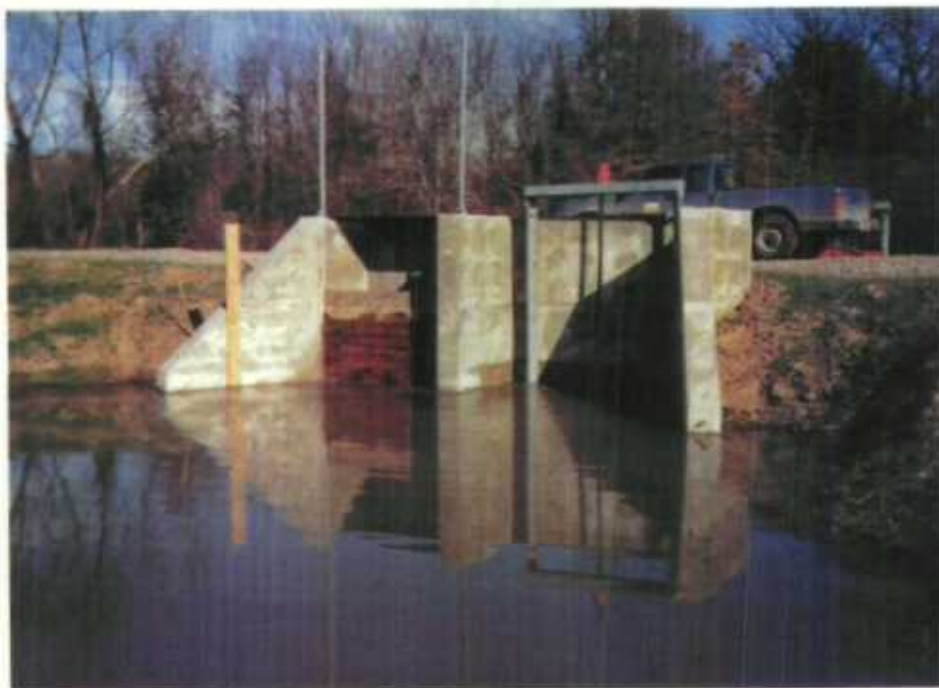
Finished twin 72-inch structures in the main levee of the Dixie Unit. In this picture the structures are holding out a large flood, while holding a smaller flood in the sloughs and impoundments on the Unit.
