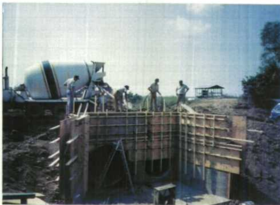
Second concrete pour on the Cache Bayou side of the twin 72-inch structures on the Dixie Unit.
