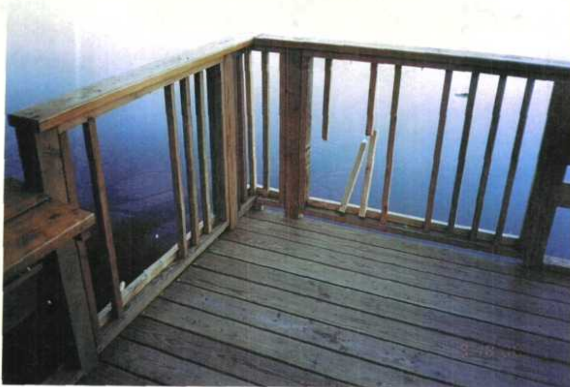
9/18/00 Print 01-1-8 GRM Vandalism on new pier by kicking out the 2X2 pickets.
