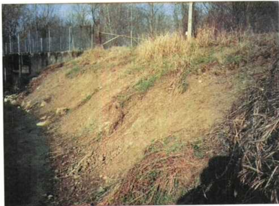
3/8/00 Print 00-1-2 GRM Sod dug up by nutria feeding on grass roots on levee between boathouse and lake WCS.
