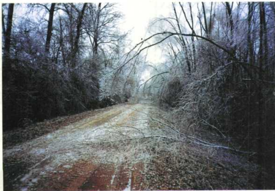
12/14/00 01-1-11 GRM Ice storm damage along Levee 1 from the December 13 storm.
