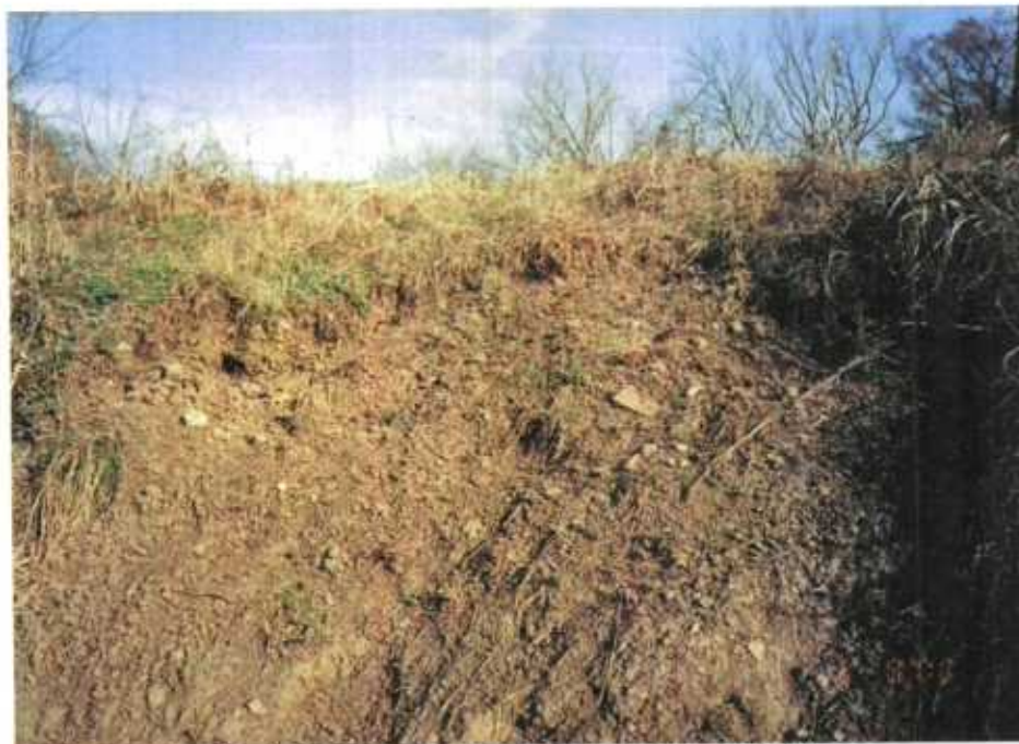
3/8/00 Print 00-1-3 GRM Sod dug up by nutria feeding on grass roots on levee between boathouse and lake WCS.
