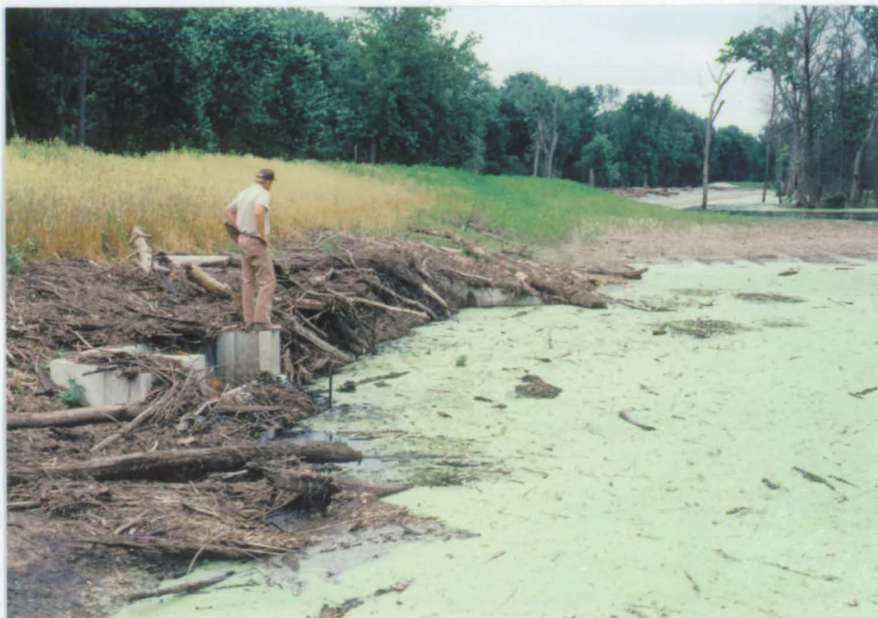
As floodwaters on the Clarence Cannon NWR recede in June, temporary Tractor Operator Alan Lagemann ponders the cleanup work ahead. Above, debris collects at the outlet structure. Note debris on spillway in upper right background. See photo on page 7 to see what the outlet structure looks like under all this debris.
