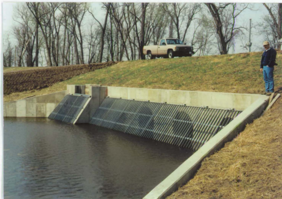
In May, Chief of Refuges Rob Shallenberger visited the refuge. Above, Rob looks over the newly completed outlet structure adjacent to the Mississippi River.
