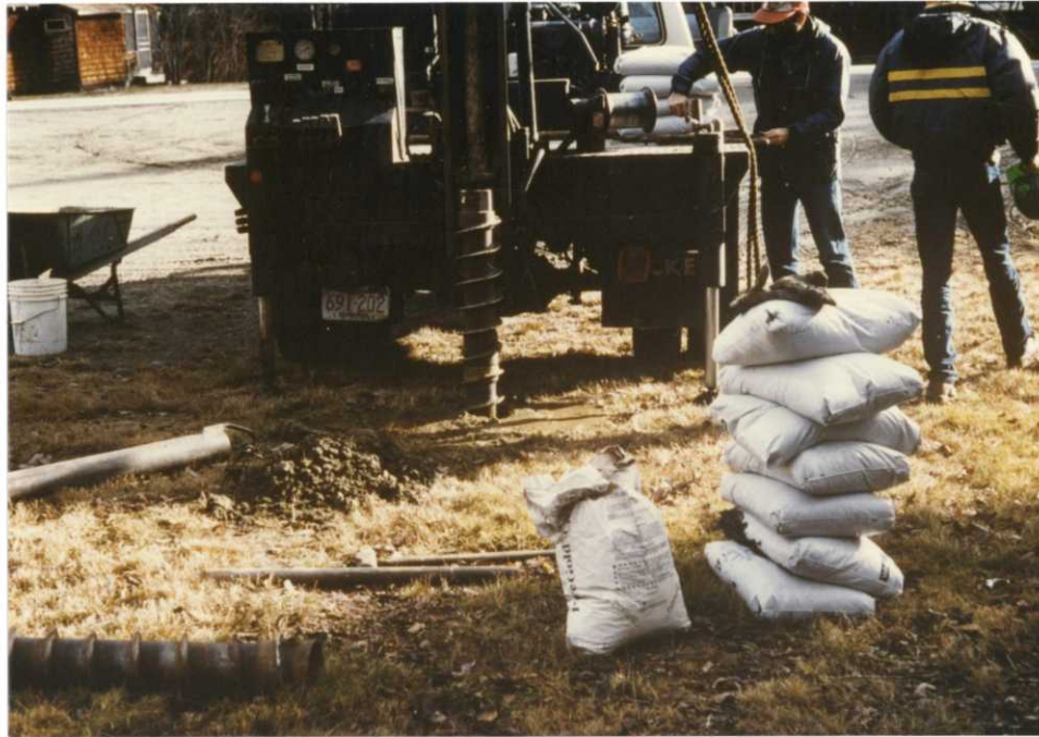
Three wells were installed to monitor underground water contamination.
