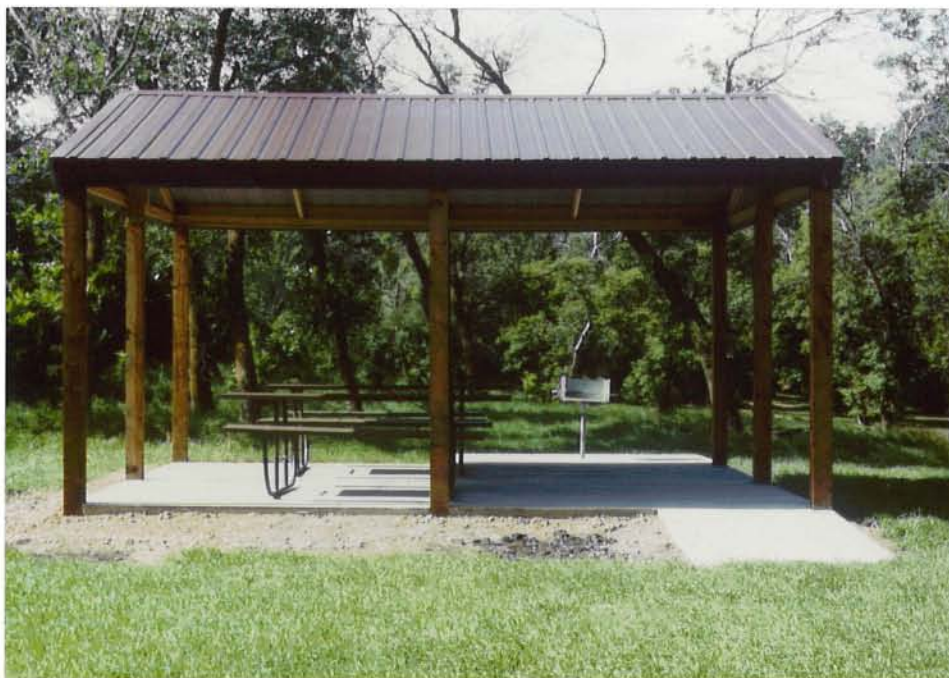
The new picnic shelter offered more accessible opportunities for the public. KLA
