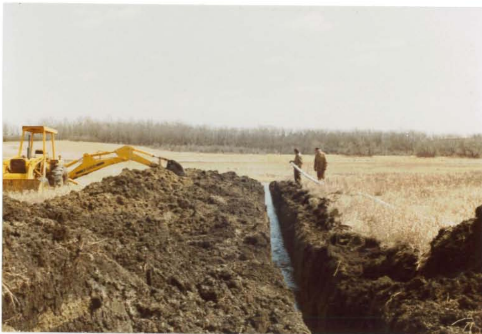
Rob Hoflen and Chris Schuler backhoed a trench and gravity flowed water to fill two small and one larger dry wetland (beyond road). A 4" PVC pipe with control valve was installed for use when water is needed in the future. (Refuge residence in left background and shop in right background.) 4/83 - DGP
