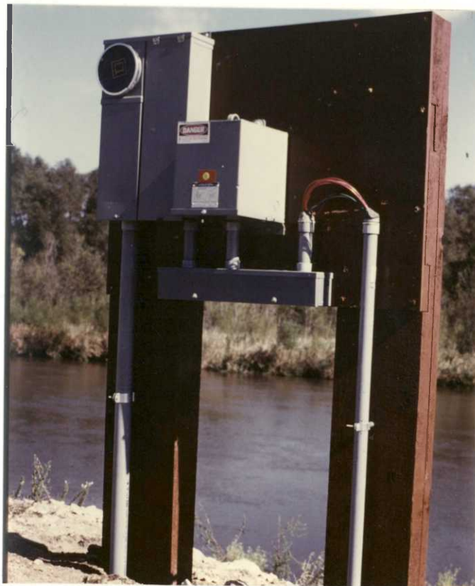
Electric fish weir panel with a portion of the controls in place.
