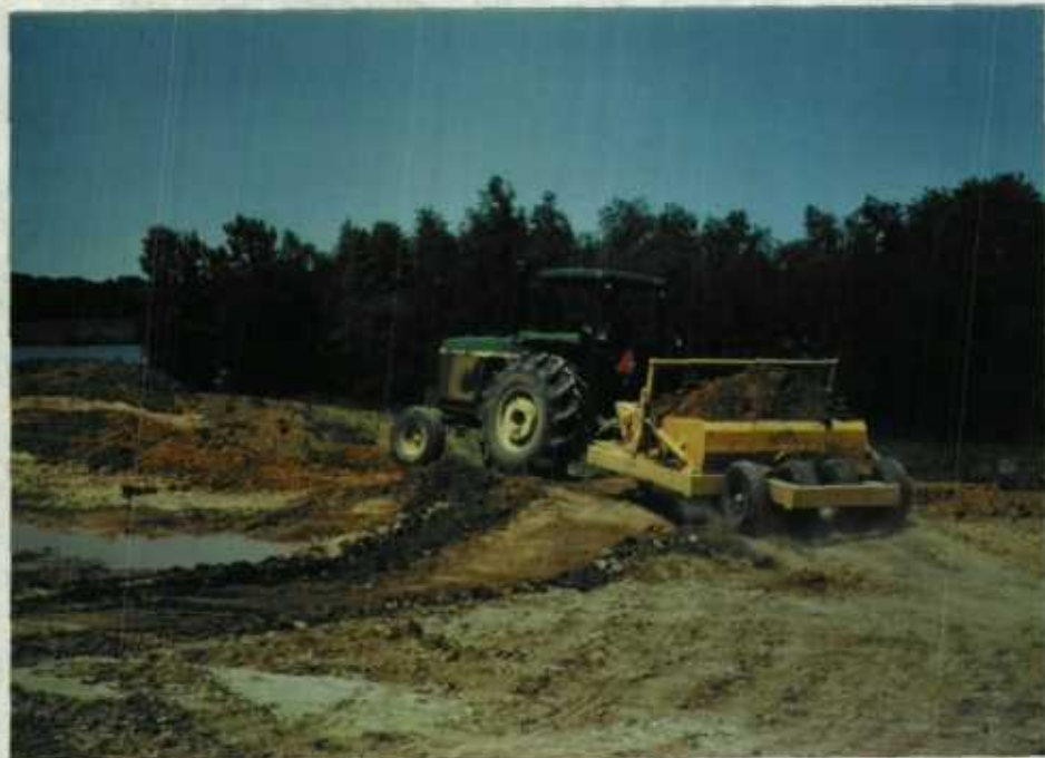
80-8-11. All of the earth moving and heavy equipment was provided by the refuge. Y.A.C.C. labor was utilized whenever possible. (LR).
