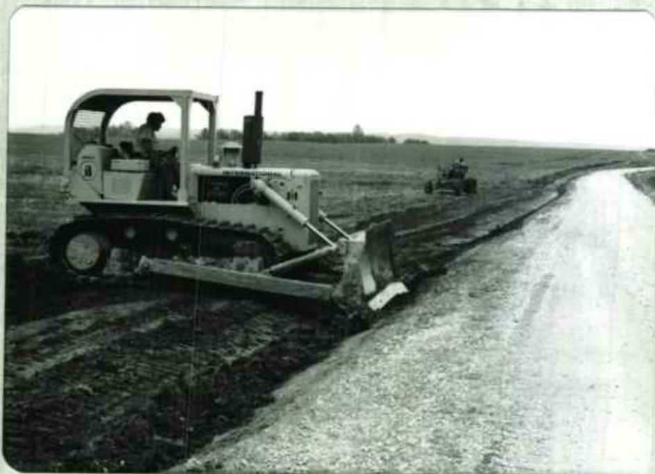
R3-17-80. The Sulphur Well peninsula road was reshaped and ditched in connection with the terracing work in adjacent fields. (LR)
