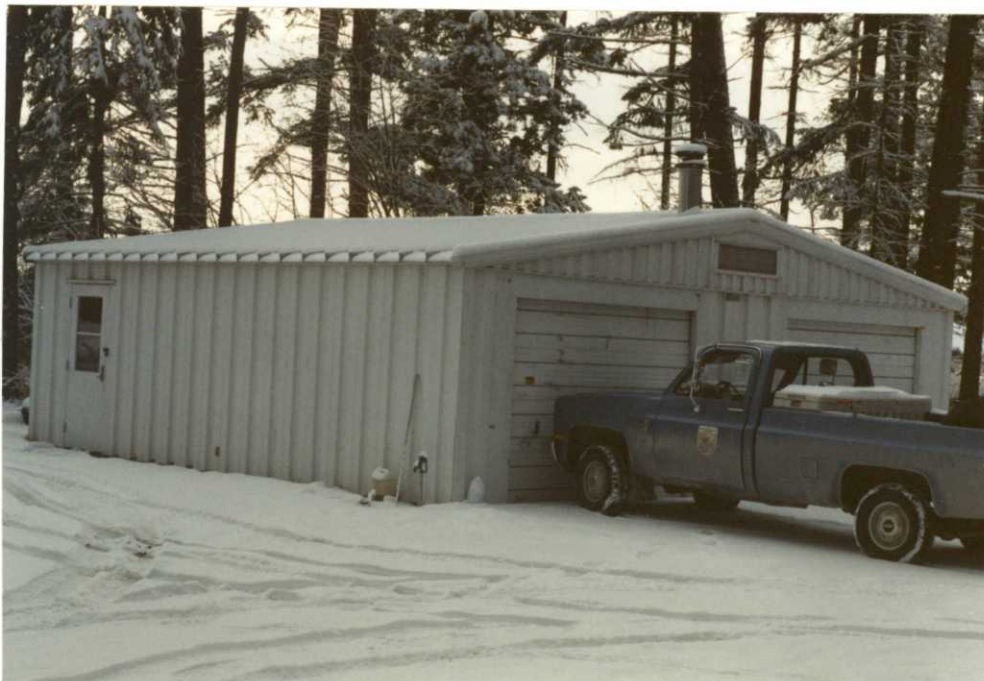
Figure 14. The building was put up by force-account. Work was slowed due to weather delays, other duties and trying to remember how to "put it back together". Most of the insulation, electrical work and wood stove installation was completed by late December. R.W. 12-19-88
