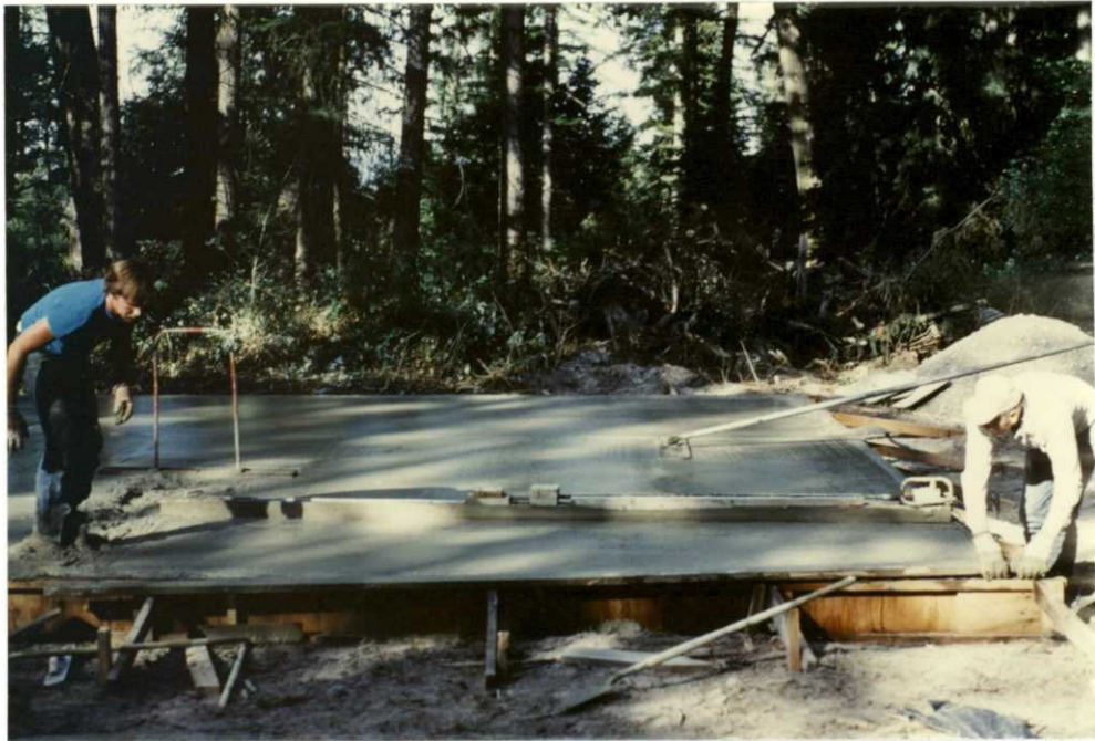
Figure 13. A site for the "new" shop/storage building was selected behind the administrative office at the Hatchery complex. Several large spruce and larch trees were removed in early August. By mid-month the contractor had completed the concrete pad. K.S. 8-16-88
