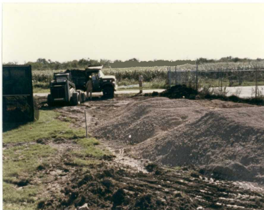
Before -- In the beginning, maintenance workers prepared the pad. Mancha reaches into the cab; Maxwell supervises. (NO84, SA002-14, JI)
