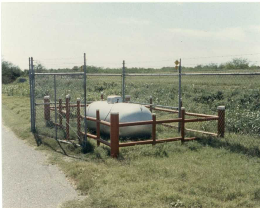
Mancha built this sturdy barrier around the greenhouse's bottle gas tank to protect it from straying vehicles. (21MR86, R4-03, JI)
