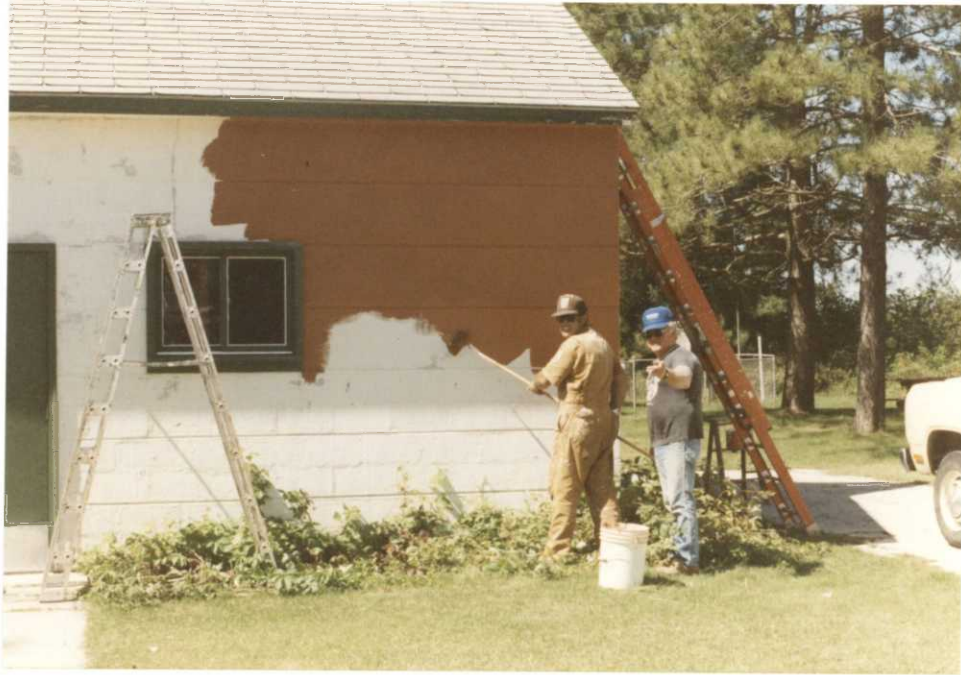
Figure 25. A fresh coat of paint on the old eyesores completed the transformation. MGT
