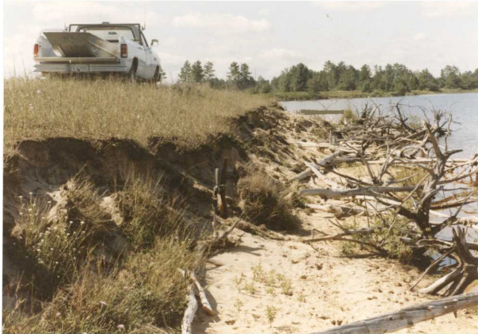
Figure 9. The Marsh Creek dike, created in the 1930's and 40's, is losing the battle with high water. Fortunately, most refuge dikes are in far better condition. DAF
