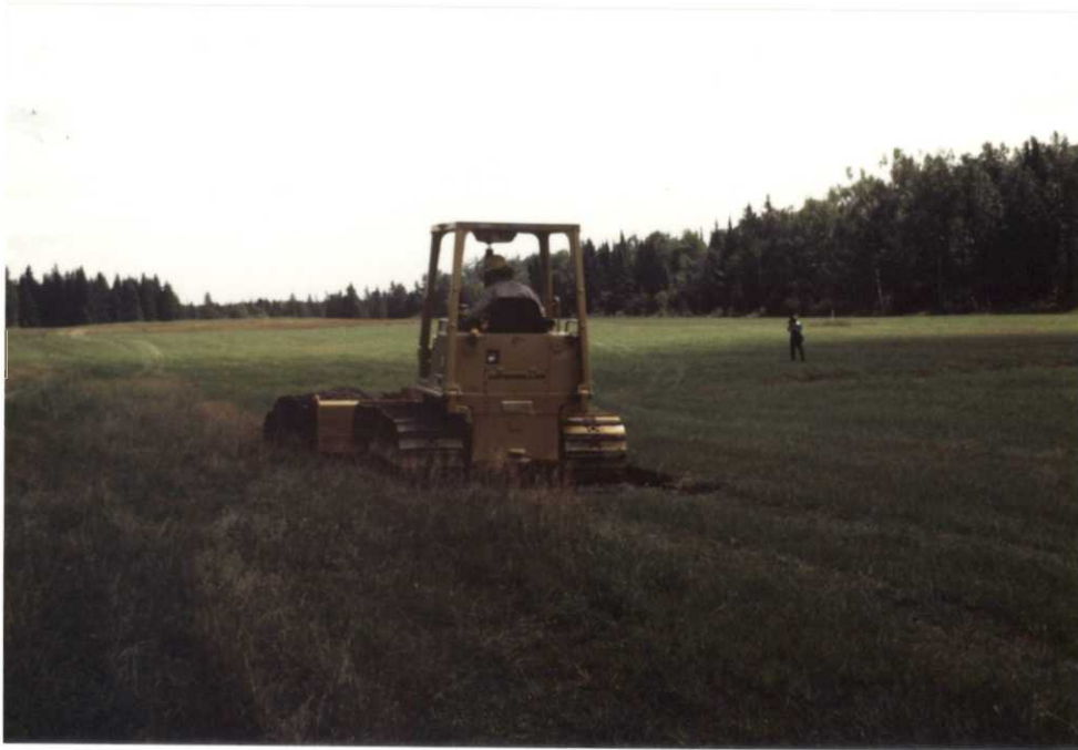
Maintenance Worker Huhta begins a wetland restoration on CRP acreage in St. Louis County... 8/8/88 JWF
