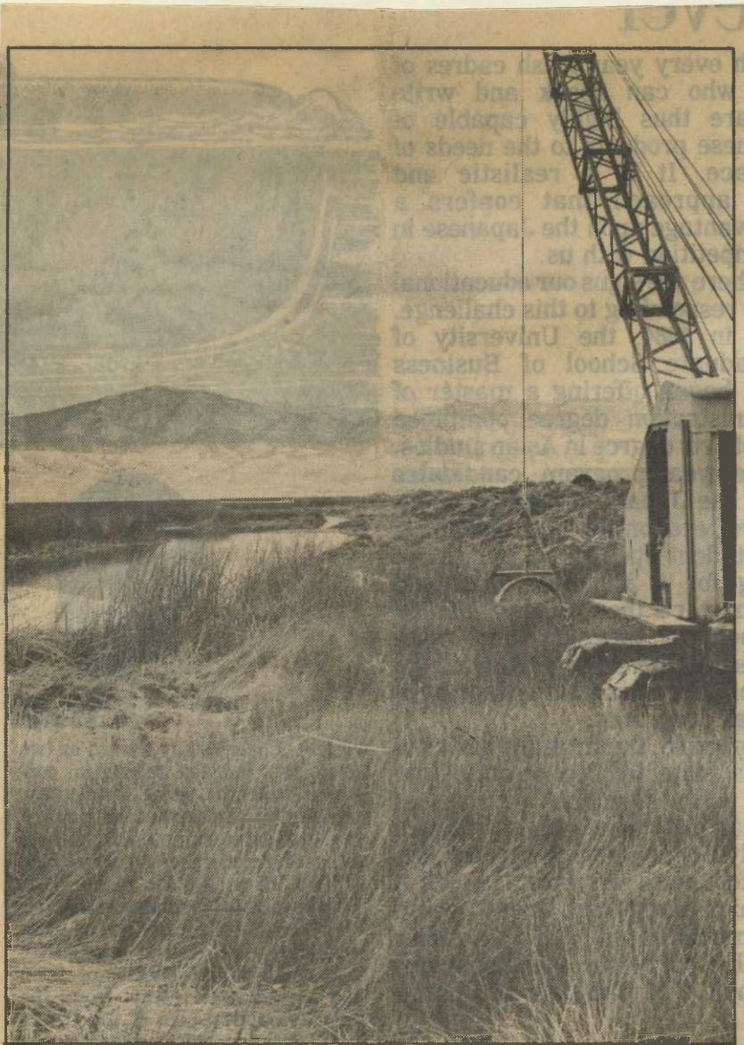
Draglines recently completed the dredging phase of an extensive improvement project at the Ruby Lake National Wildlife Refuge. Lacey Construction Company of Cascade, Idaho, spent several weeks dredging 83 "fishholes" in diked units at the refuge and digging channels that will facilitate water management at the Ruby Marshes. Story and additional photos appear on Page 4.
