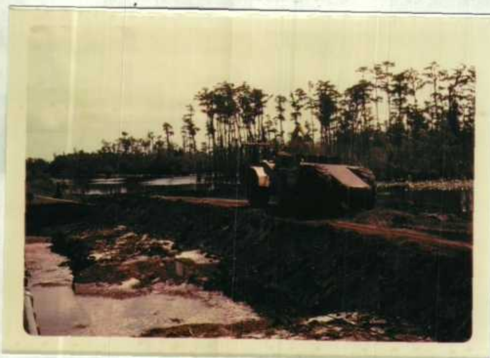
A hurried-up coffer dam was constructed after the No. 1 Sill Structure collapsed and swamp started loosing water at a rapid rate. NS-28-77, JRE.
