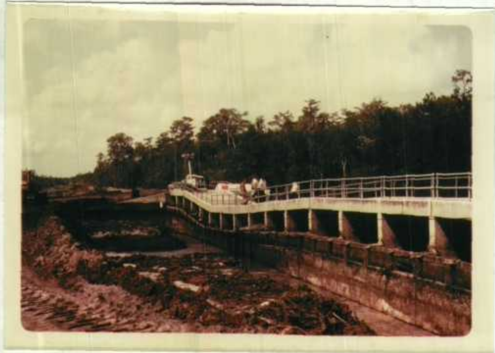
A sagging Sill structure. NS-26-77, WDM.
