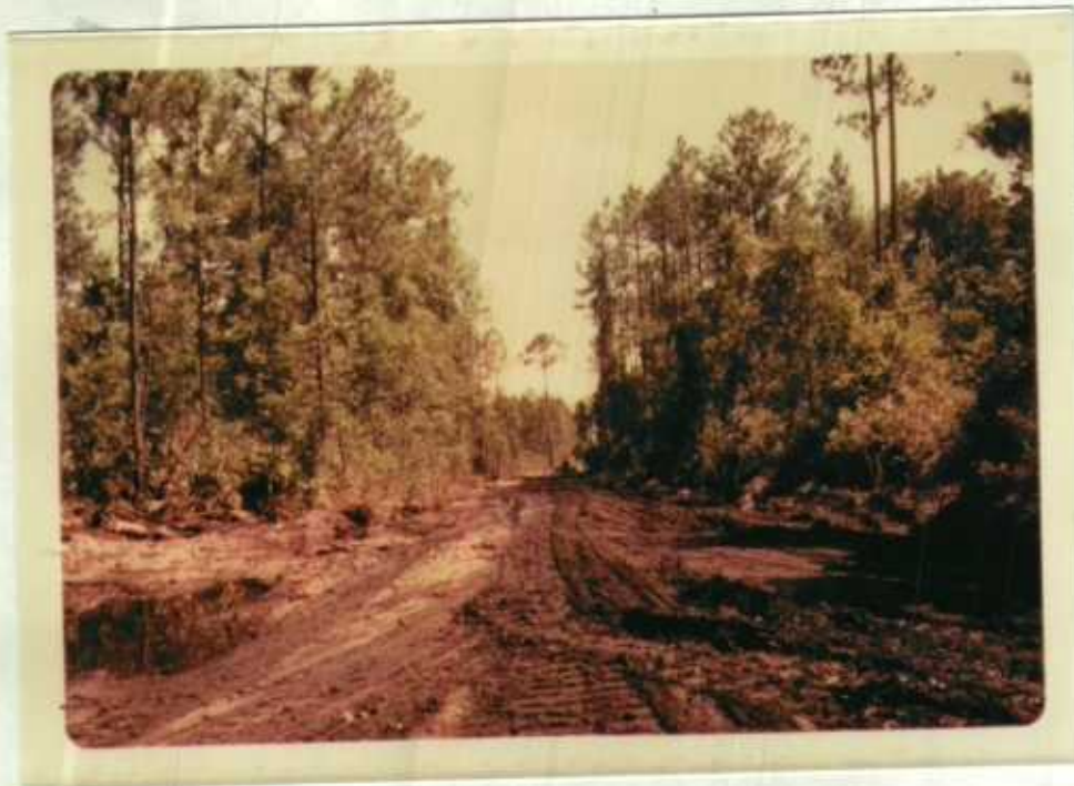
Road work is a continual chore. This is Phernetton (Refuge Forester) Phreeway. NS-25-77, Staff.
