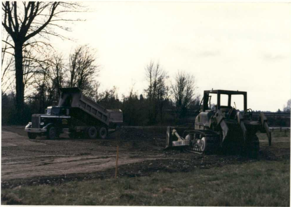
Figure 30. Fill for the parking lot was brought in from a local gravel pit while Bill Schaff ran the dozer. EH-88
