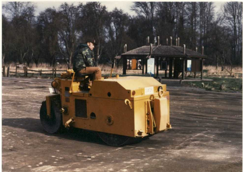
Figure 31. Bob Watson makes sure the parking lot is packed and FLAT! EH-88
