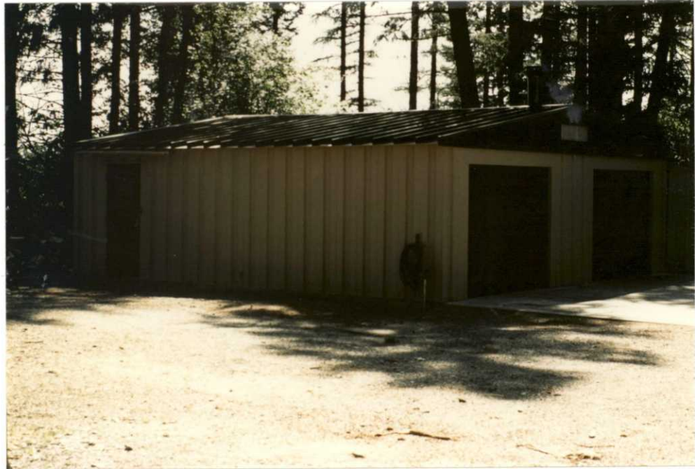
Figure 24. The shop building after painting. The new paint improved the appearance of the building, as well as conforming its appearance with other buildings at the Fish and Wildlife Center. PG 8/20/91
