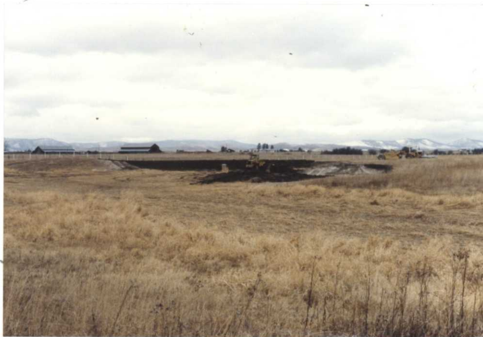
Figure 7. Construction of a dam which started in October will restore this 15-acre wetland. An aerial view (next photo) also shows the wetland more clearly. JM 10/91
