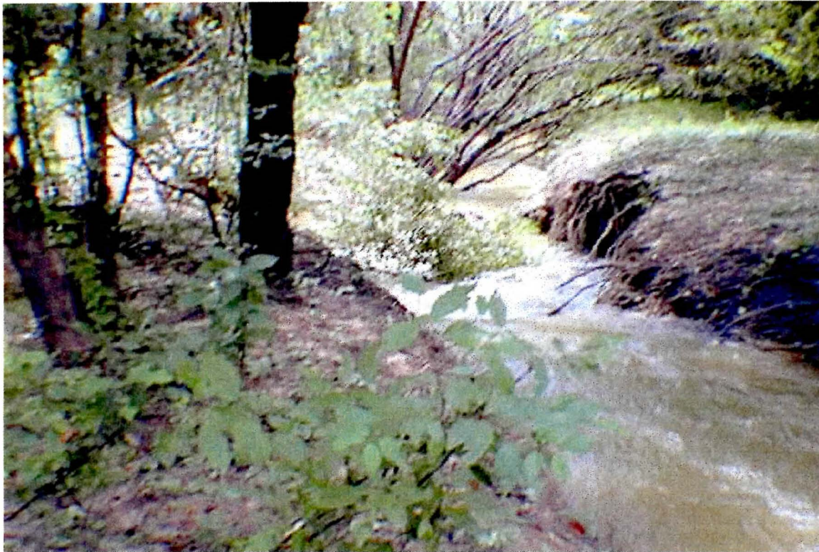
The washout at Steep Bank Creek; UO-97-1; 7/97; MS
