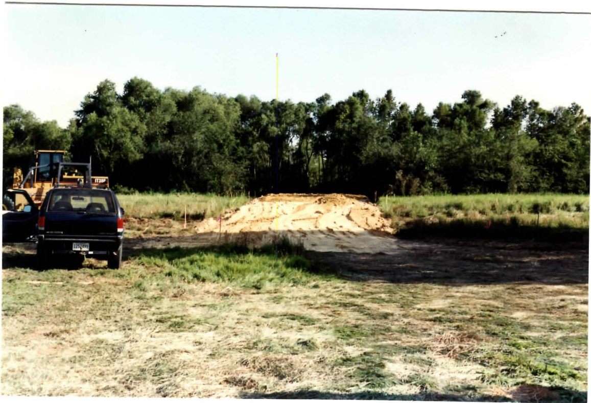
Construction of earth ramp leading to Black Bayou Lake fishing pier site. LWD97-8; 10/97; KO
