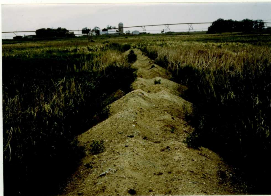
Burns Easement (44X) Pope County, filling violation where a farmer placed earthen fill to enable his center pivot irrigation system to cross the wetland. 81-15 DEM
