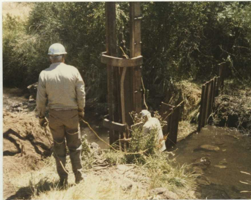
Clyde Miller and Norm Warneke installing piling in the East Canal to improve irrigation in the adjacent field.
