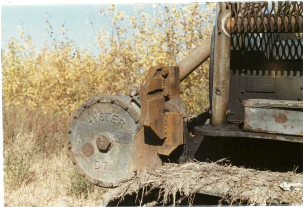
Closeup of ROPS support designed by welder. This section moved two inches while testing. Correspondence with Pennington stated the D-7 met the test at the point of bending. He will return to straighten support and certify the machine. (R-970, P-19, TSS) (10-29-84)
