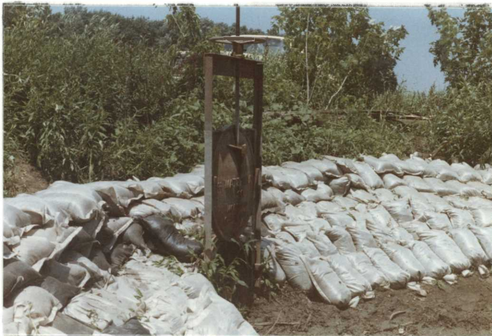
Erosion control of water control structure located in transport ditch. (R-967, P-19, TSS) (06-28-84)
