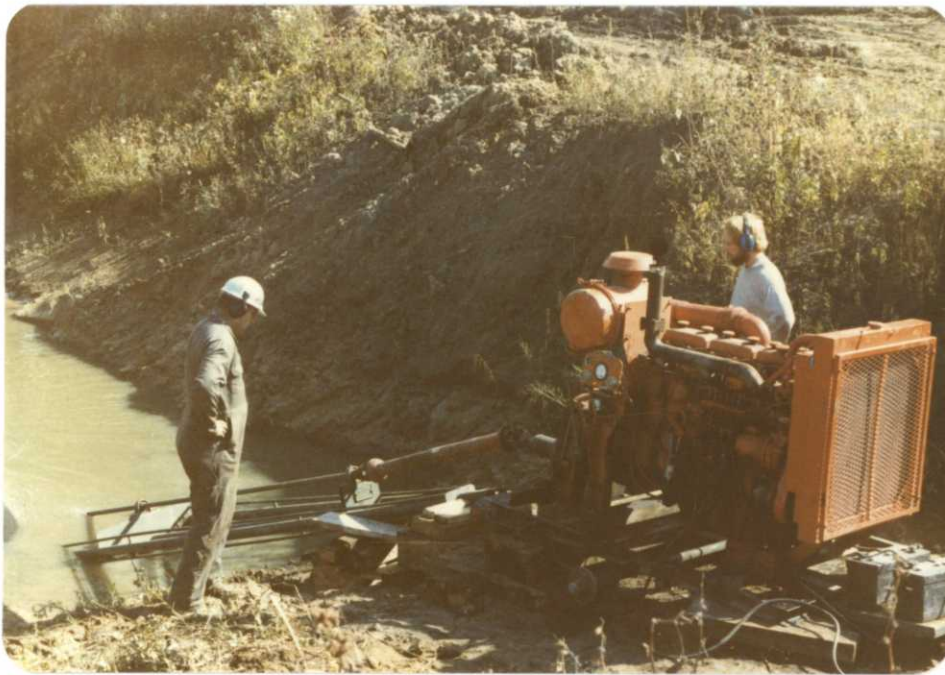
Bill Watts, maintenance worker, and Kevin Kenow, manager trainee, are checking the Waukesha diesel motor and Crisafulli pump for vibration. (R-931, P-17, TSS) (10-3-79)
