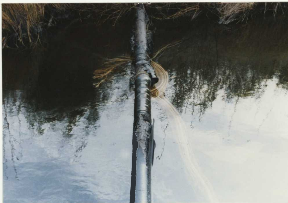
FIG. 10. ONE OF SEVERAL OIL SPILLS (LEAKS) WITHIN EXXON'S CLAM LAKE FIELD. OLD FLOW LINES (ABOVE) ARE BEING REPLACED AND PUT ABOVE GROUND TO MONITOR MORE EFFICIENTLY. (AA)
