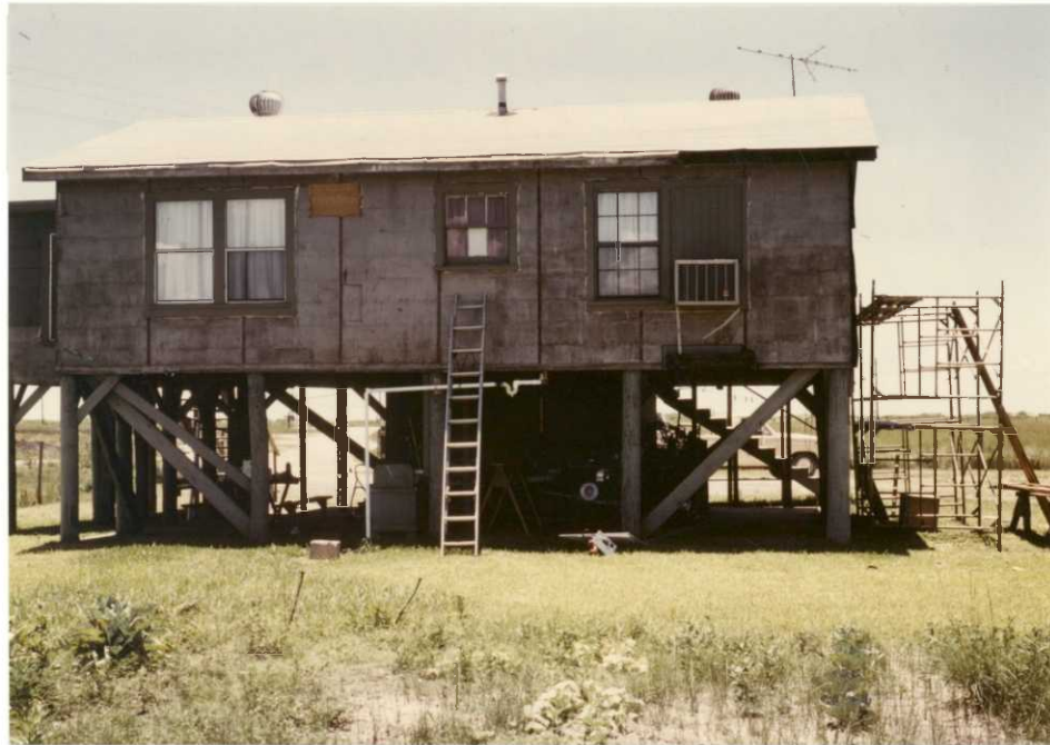
THE REFUGE RESIDENCE WAS IN NEED OF MAJOR REHABILITATION AS IS DEPICTED IN THIS PHOTO TAKEN BEFORE WORK BEGAN 84
