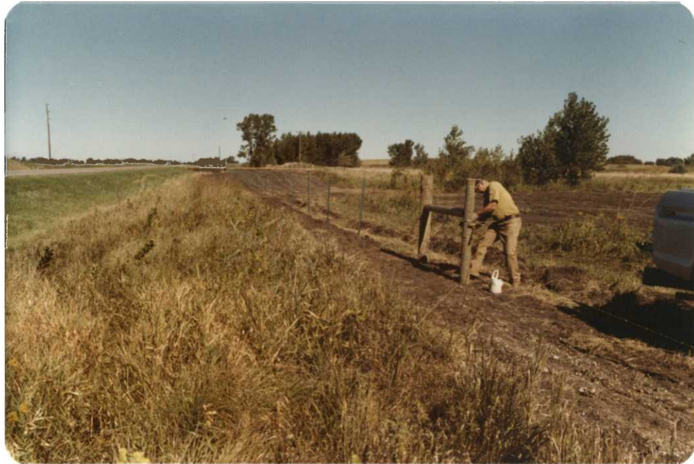
Figure 8. Harry Jones constructs new fence on the Payne WPA in Lake County. 80/32-18a 9/10/80 BTS
