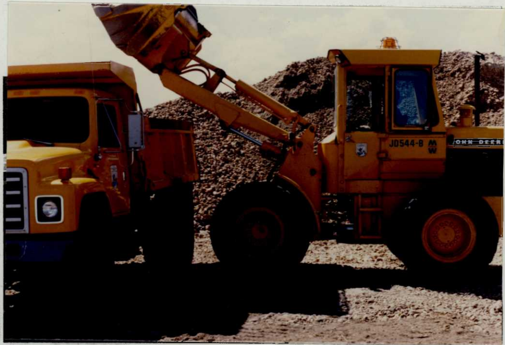
A few days' work was necessary to repair an access road near the Moen WPA.
