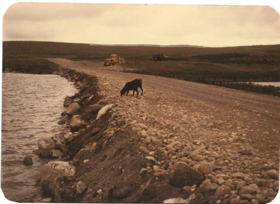
Riprapping Iverson Dike included widening the north slope with large gravel. . . June 1976 F.W. Cameron
