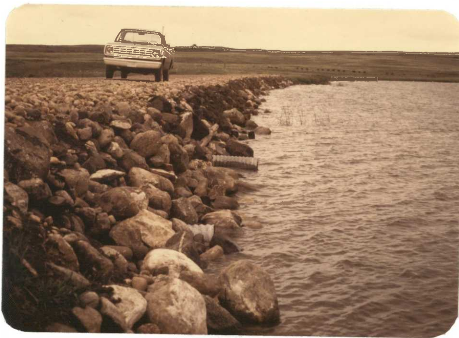
and then adding boulders, especially around the two culverts. June 1976 F.W. Cameron
