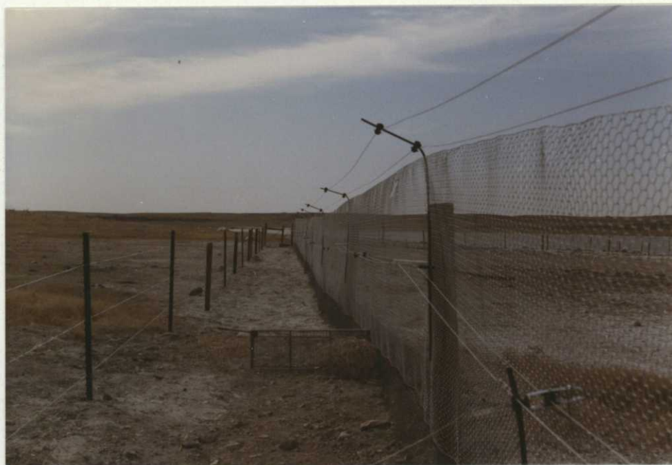
Photo 35. Completed electric predator barrier fence with cattle fence to protect from cattle on adjacent private land, West Island WPA, 6/85 - LDW.
