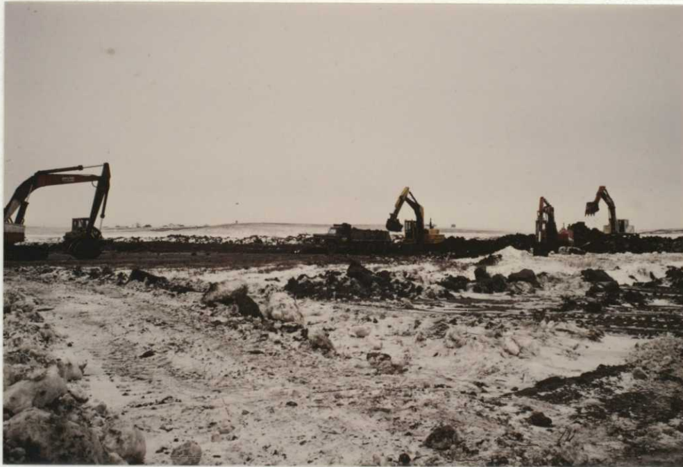
Photo 37. DU project with large selection of equipment digging trenches and filling trucks for nesting islands, Brinkman WPA, 12/85 - RAH
