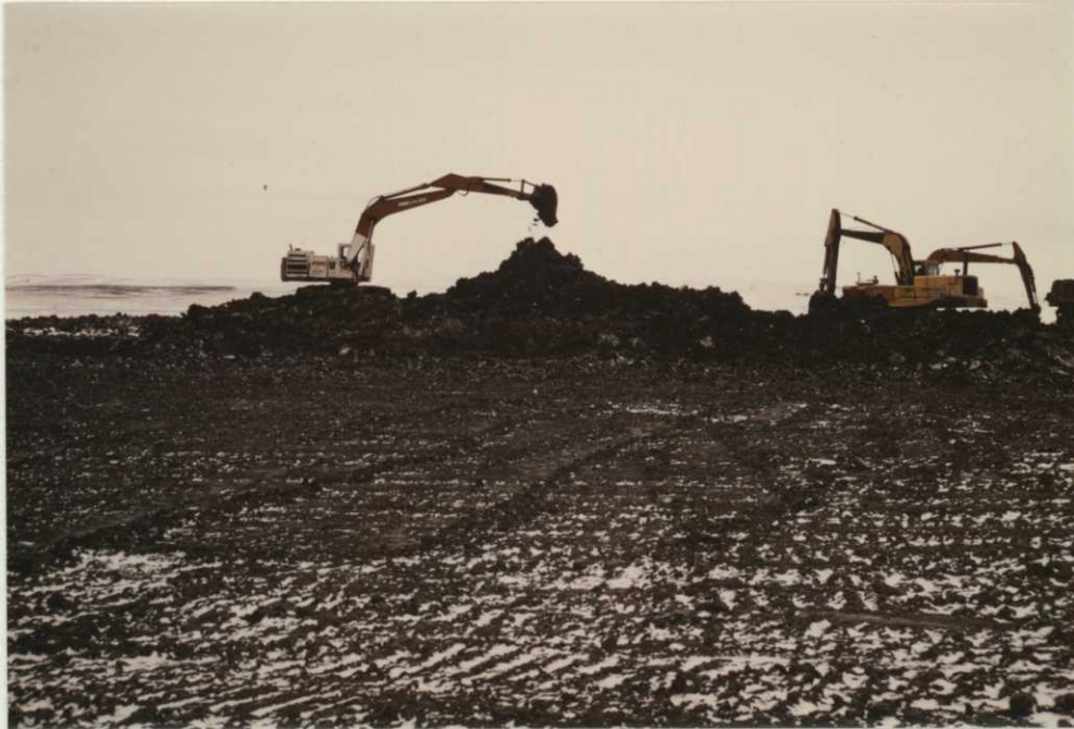
Photo 36. Ducks Unlimited (DU) contractor digging peninsula cut-off trench in frozen lake bed at the Brinkman WPA, 12/85 - RAH.
