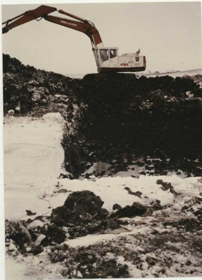
Photo 39. Construction was often difficult and messy when various natural springs were encountered during excavation of peninsula cut-off, note standing water at 10-15 o below temperatures, Brinkman WPA, 12/85 - RAH.
