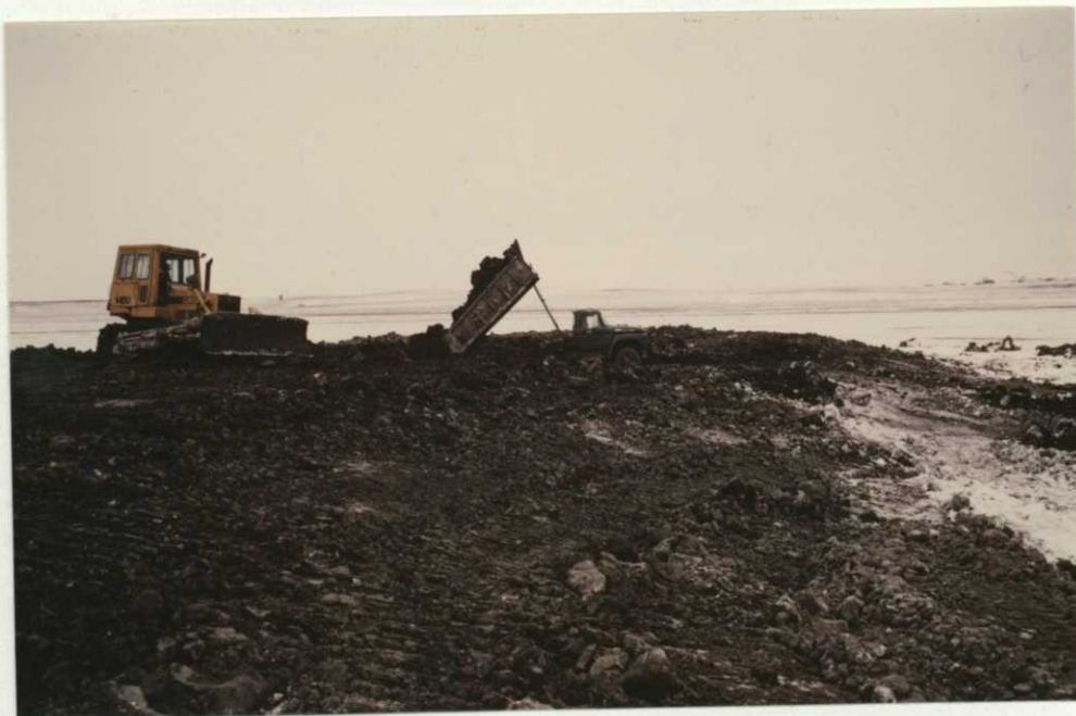
Photo 38. Adding fill to nesting island in frozen lake bed, Brinkman WPA, 12/85 - RAH.
