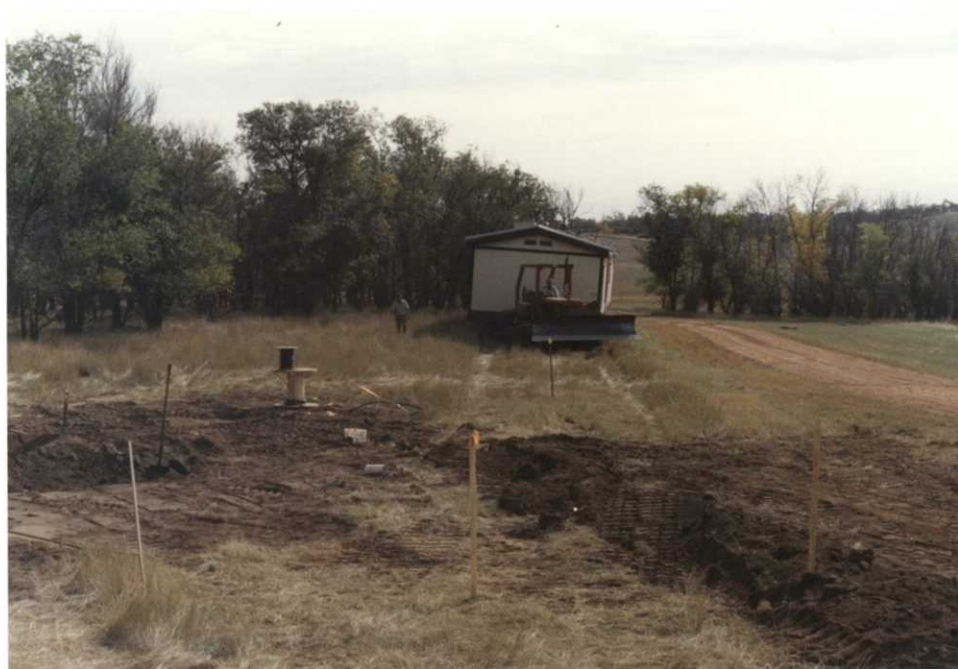
Duane Brenneise pulling the bunkhouse into place with the dozer. Brian Mautz walks along to help guide him into place. 9/92 DJB
