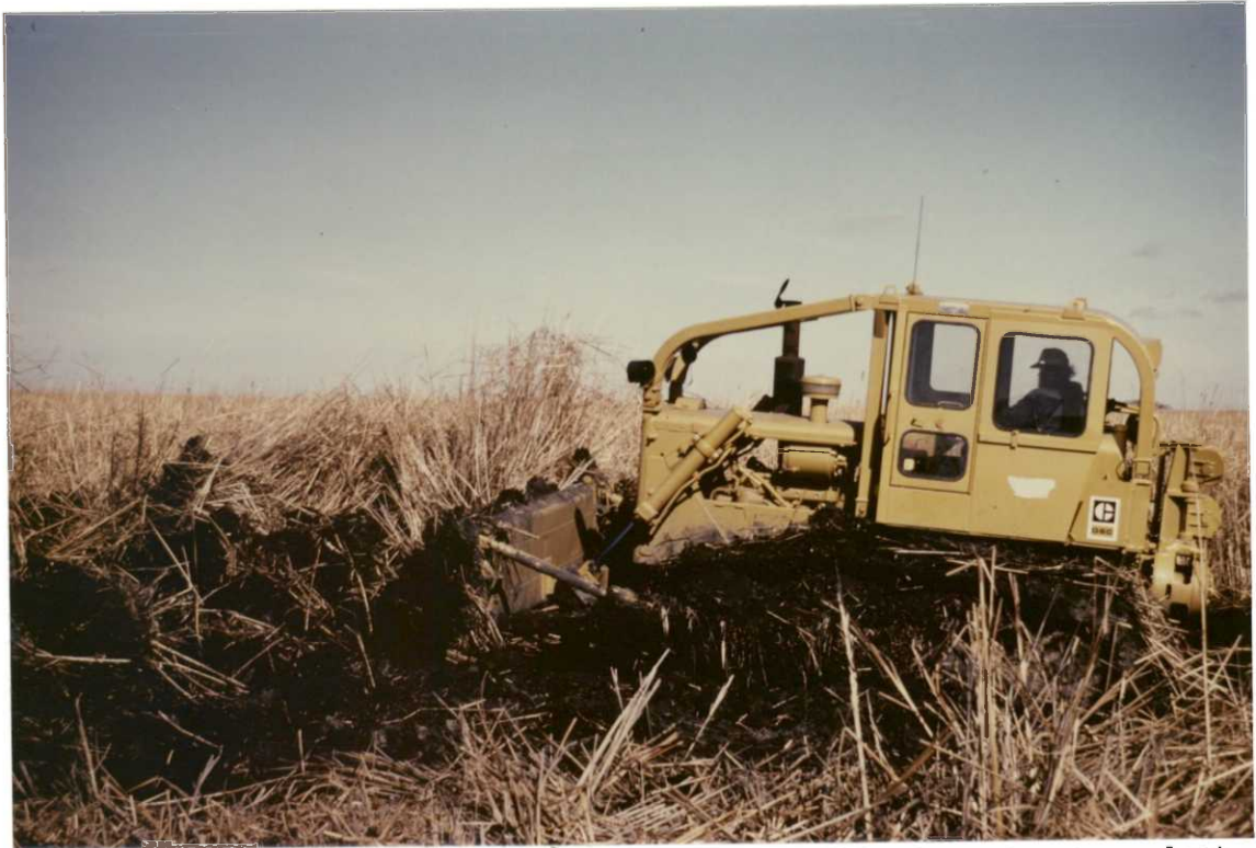
Initial stages of island construction, Alice WPA, Cass County. Just as important as providing safe nesting areas is the creation of open water areas in cattail-choked marsh. LAJ-1984
