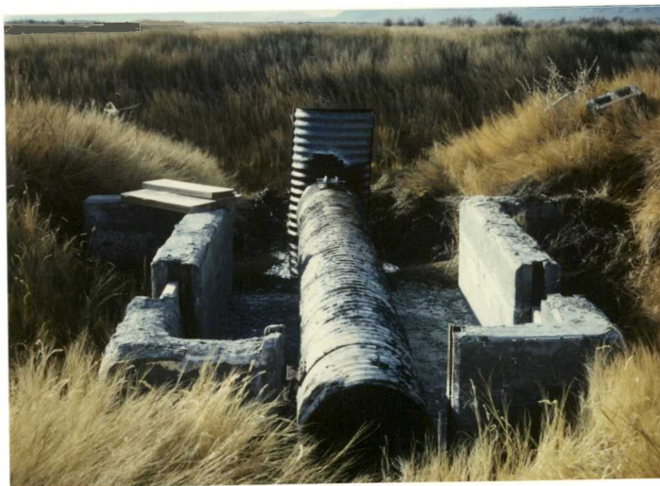
This culvert was installed in Gadwall Unit to replace the non-functional concrete stop log structure
