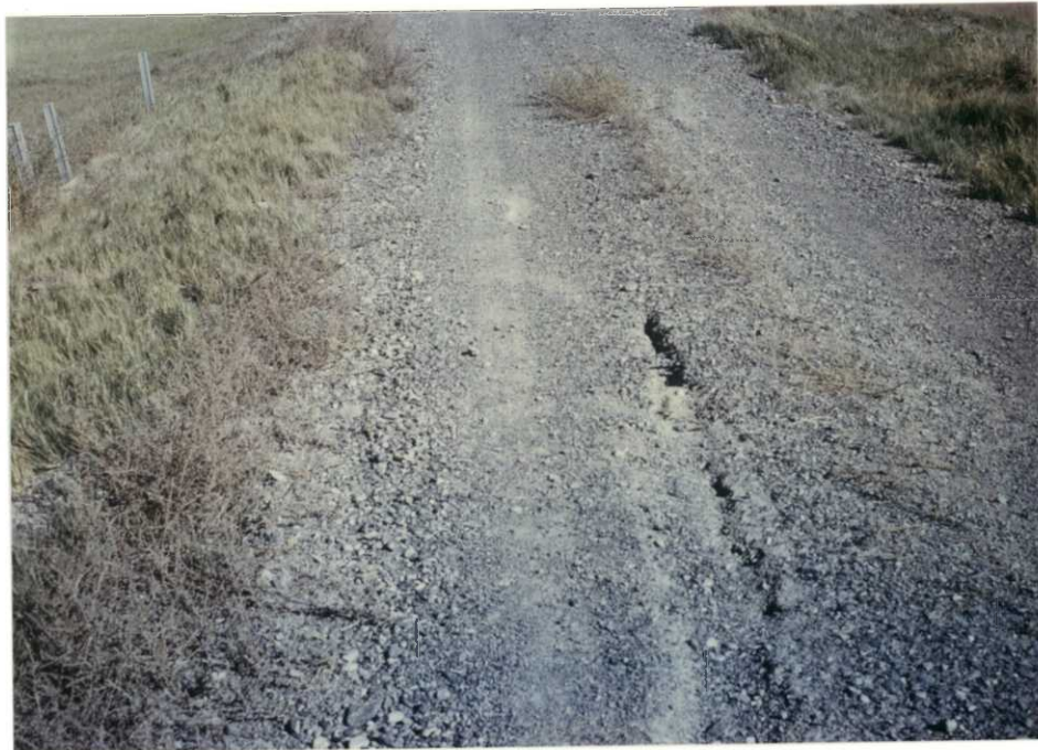
This 50' long X 6' deep crack resulted from the 1.5 years that the two adjacent units were dry
