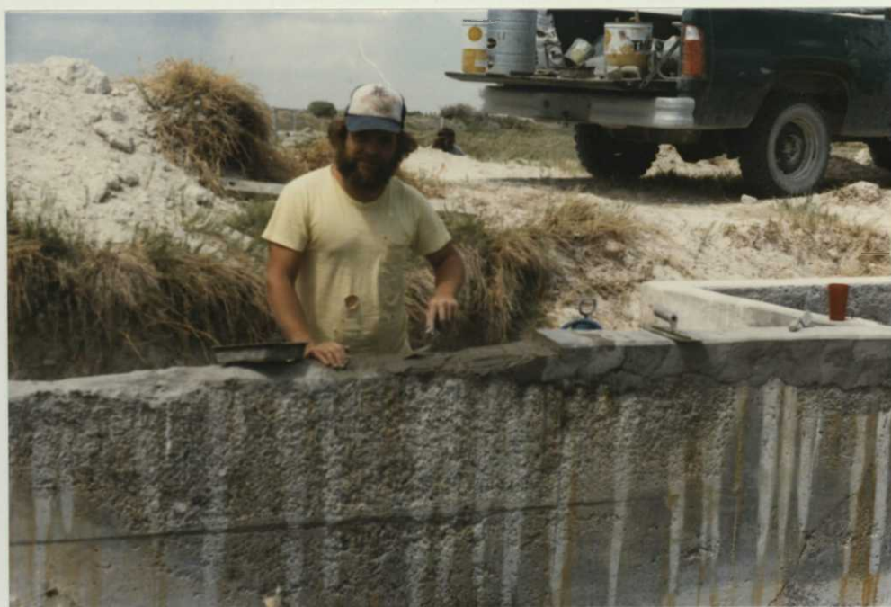
Fig. 14. 8/26/85 Raymond Timm works on other side of structure C-5. Thorite was applied in layers and required fast work in hot temperatures. CRD
