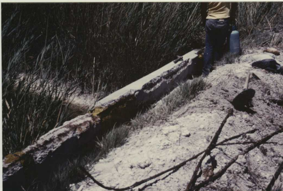
Fig. 12. 1003.053 7/30/85 WCS C-1. Extensively rusted rebar was removed. Other exposed rebar was cleaned with acid before rebuilding the eroded sections. CRD
