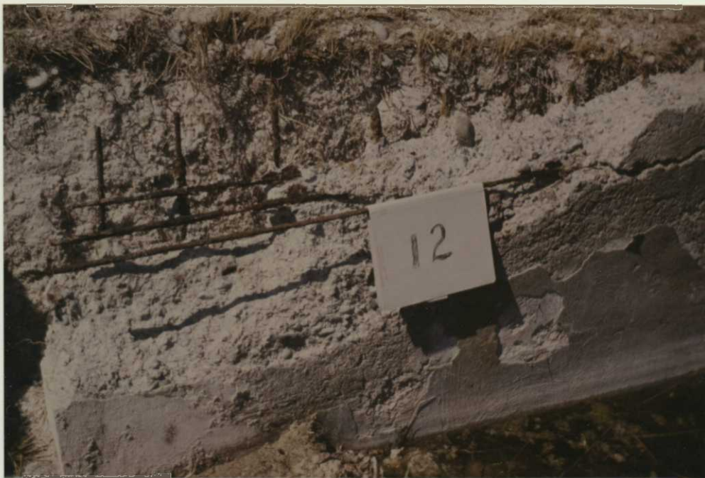
Fig. 9. 1003.042 2/15/85 Deteriorated wing wall on WCS #12. Unmixed sand was evident in this section. CRD
