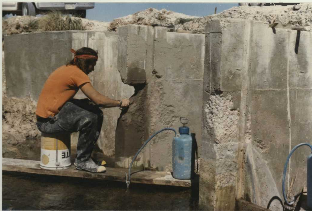
Fig. 10. 8/13/85 Bret Layland begins to fill eroded portions of stoplog slots on WCS #12. CRD
