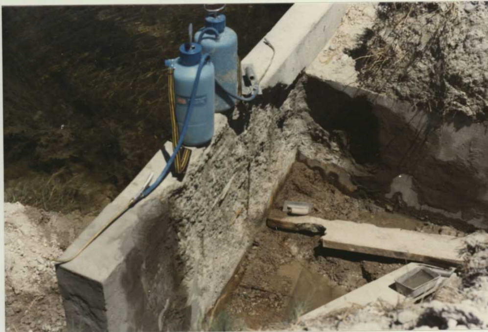
Fig 7. 6/21/85 Structure #11, deteriorated concrete below ground surface. CRD
