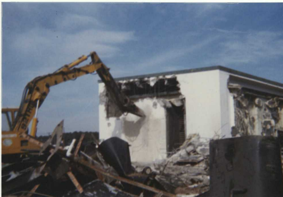
The abandoned power plant building was razed and the rubble used on the firearms range walls.
