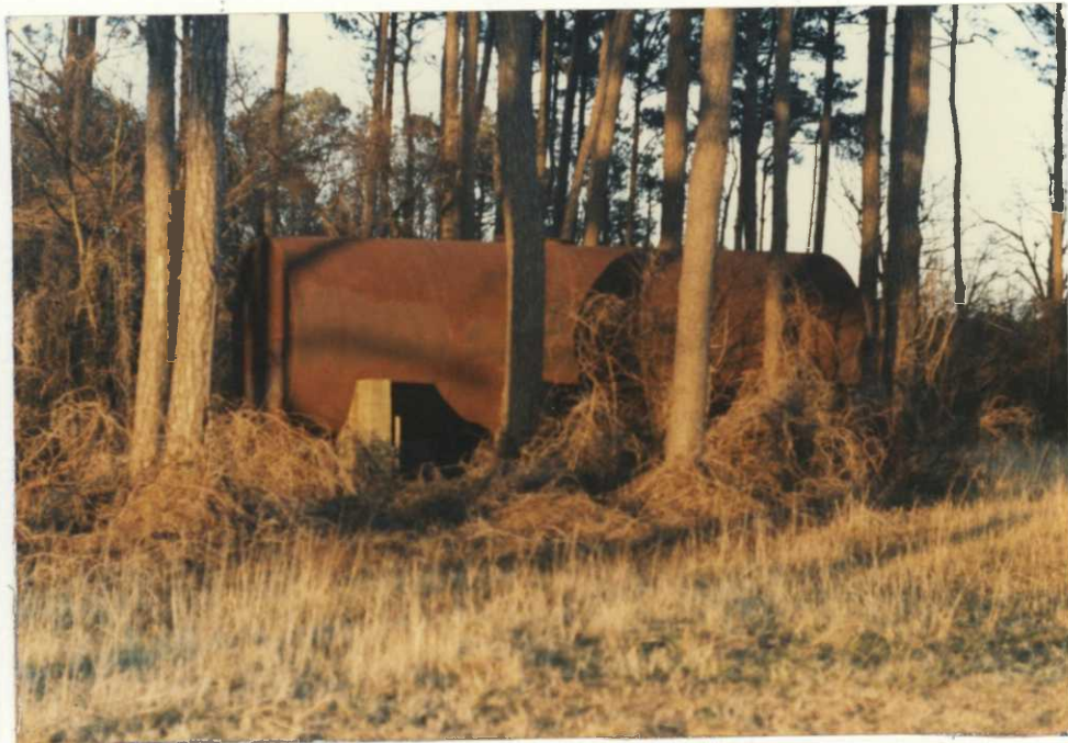
A 8 foot x 20 foot storage tank located on the future site of the new office was removed by a contractor.
