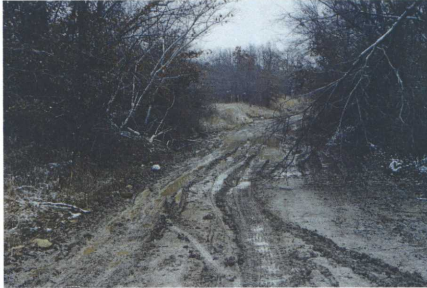
Damage to refuge roads as a result of Ice storm
