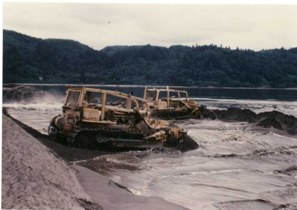
#9-Caterpillar tractors spreading dredge spoils pumped from the dredge "Oregon". Heavier sand material settles out and is secured on higher ground, while the water carrying the load through the pipe returns to the River. 89-RTV
