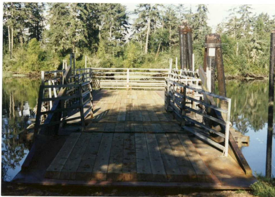
#5-A new, larger wooden deck was added to the 80-ton barge to allow for safer loading and transportation of heavy equipment using steel tracks.
