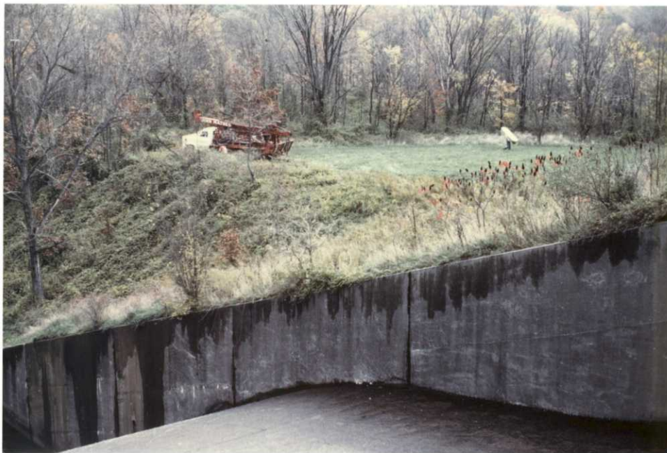
Drilling Contractors at Little Grassy Lake taking core samples of the dam to determine necessary safety modifications.
