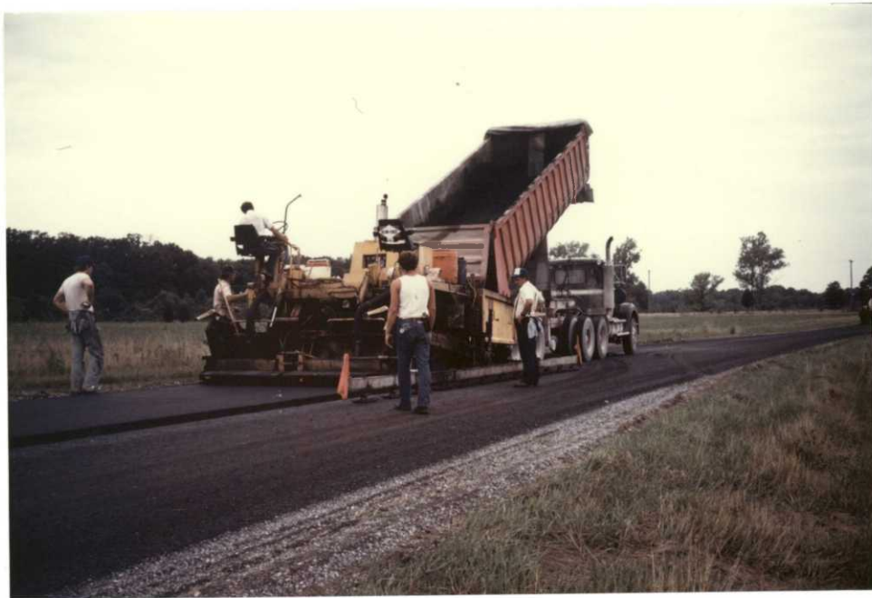
Hot mix asphalt road rehabilitation on 4.7 miles of the refuge's 28 miles of paved roads.
