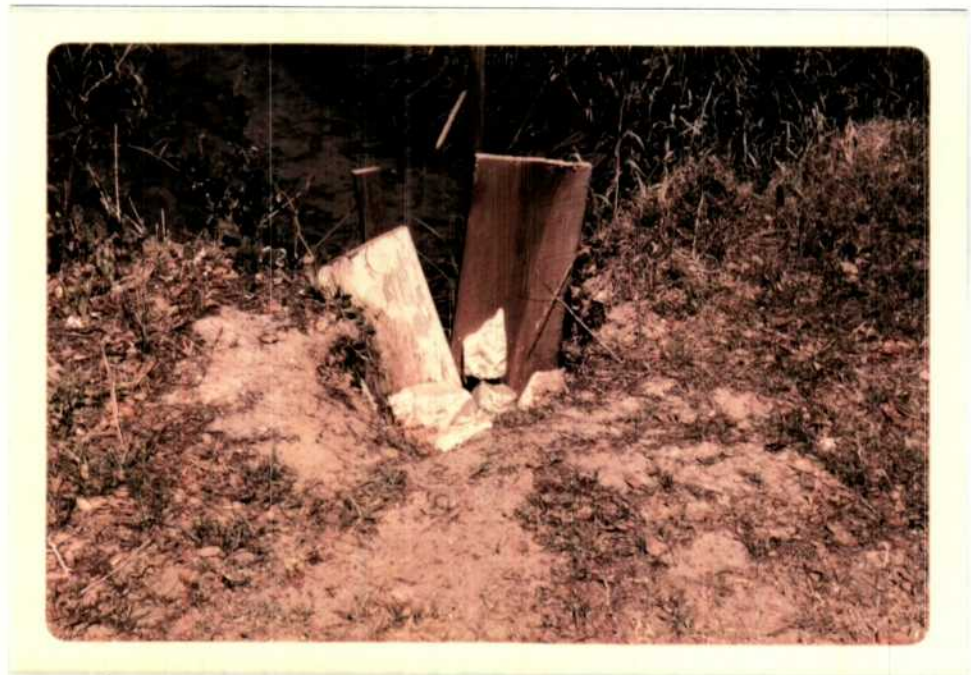
Water Control Structure? Need Rehabilitation? (Photo by Garris)
