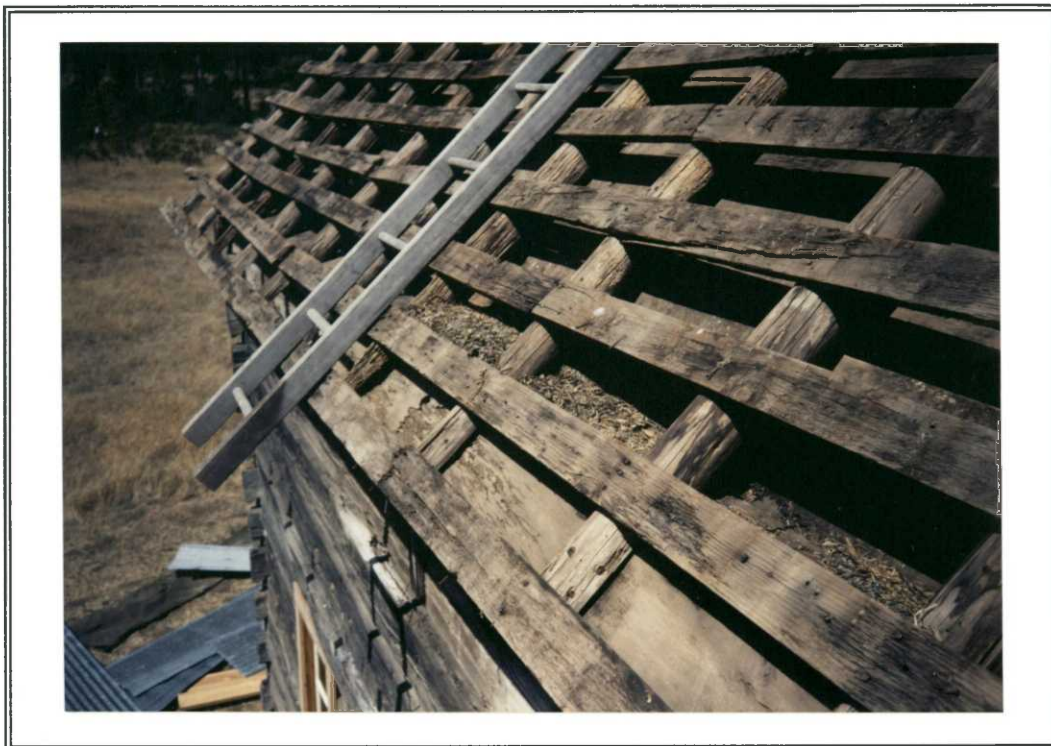
Several of these furring strips had to be replaced, but only one rafter. HC-92
