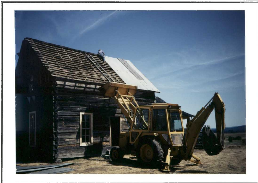
...and continues. Note old shakes had been removed prior to metal being installed.
