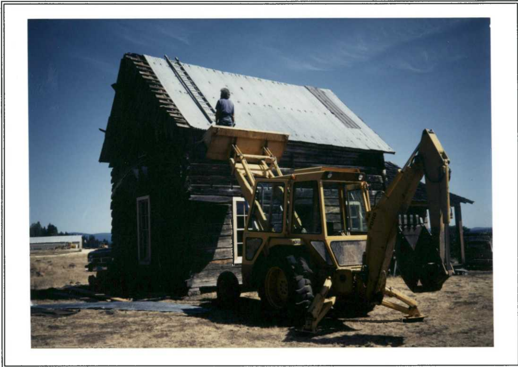
Removal of metal roofing that was placed on the south side of the cabin in 1975 begins...
