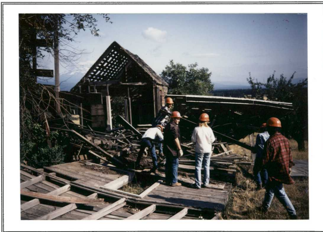
Dismantling begins; most of the building was already down from natural causes when crew started.
