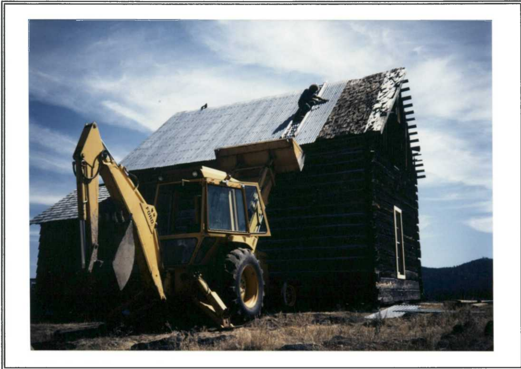
Removal of metal from north side begins (white shakes on right are sun bleached--one sheet of metal blew off last fall)... HC-92
