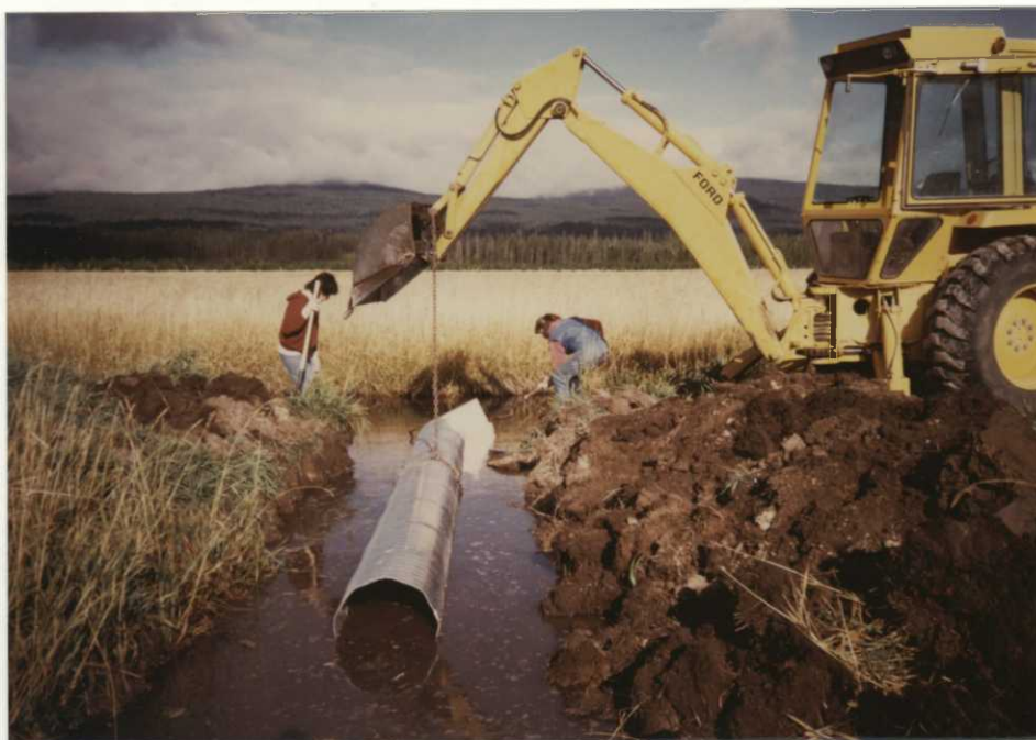
#9-WCC Enrollee's Suzanne Tyndall and Jo Ellen Lively installing a water control structure in Willard Pond dike. 86-HEC
