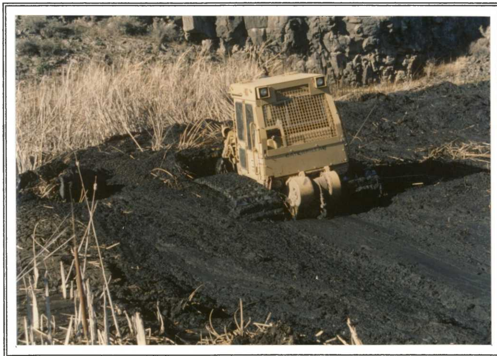
Too soft to walk, too thick to swim! The low ground pressure capability of the refuge's D-5B proved its value during rehabilitation of Marsh Unit III impoundments. 3/21/90 DEG
