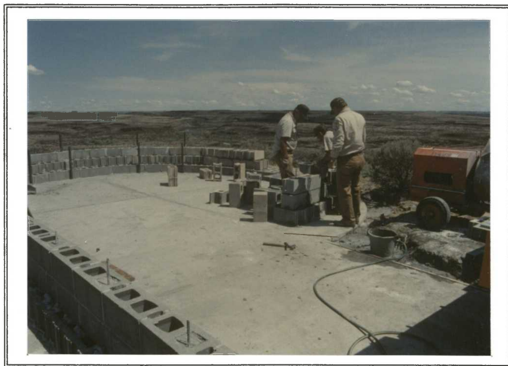
Sign supports were added and the entire structure will be faced with basalt stone masonry. 5/30/90 DEG
