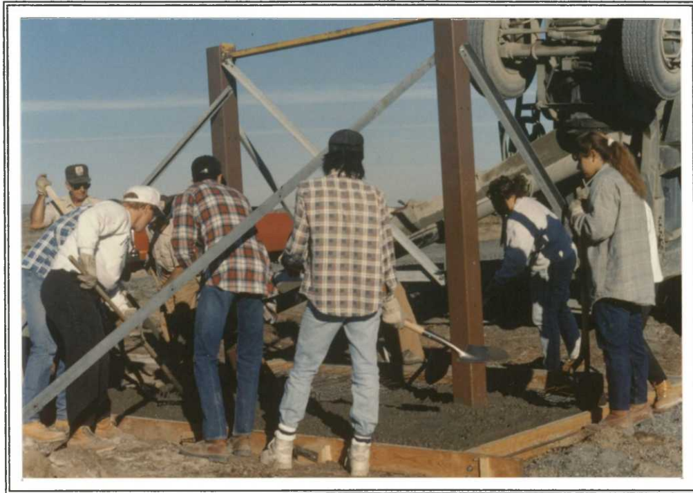
Youth Conservation Corps enrollees helped with spreading the concrete for the new covered picnic tables at the Soda Lake Campground. 6/27/90 MKC
