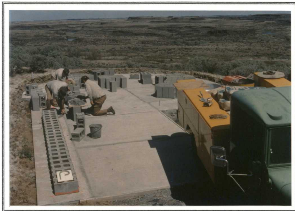
Actual construction of the Drumheller Channels NNL interpretive site finally started with construction of the block core. A clay model is visible on the first blocks. 5/8/90 DEG
