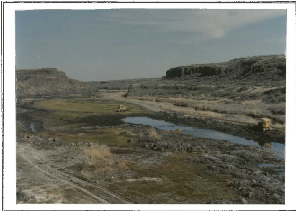
Over the years, encroaching vegetation mats nearly choked out the unit's shallow impoundments. About 1,500 cubic yards of muck and roots was removed from Pools 3 and 4. 3/30/90 DEG
