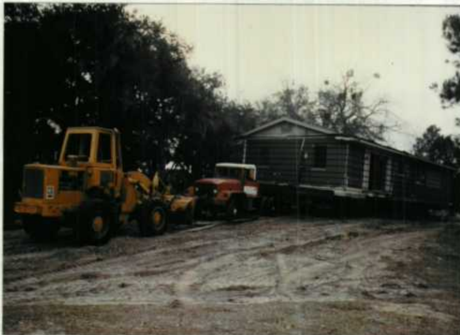
Private contractor preparing to move former private residence on Shired Island SWE-83-14 JLG
