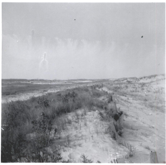
Dune Erosion Control - sand dike closing break in the dunes - sod bulldozed to give cover to dike - Old Field area -
