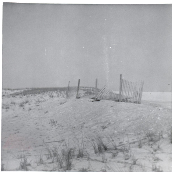
Beach Erosion Control - small sand fence and dike - note lack of sand collection -
