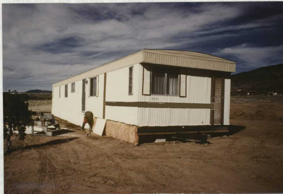
Photo 36. Joli Vollers puts skirting around the 14' X 70' mobile home we acquired surplus from the Bureau of Reclamation. It will be used to house temporary employees. 11/14/86-147, JC.
