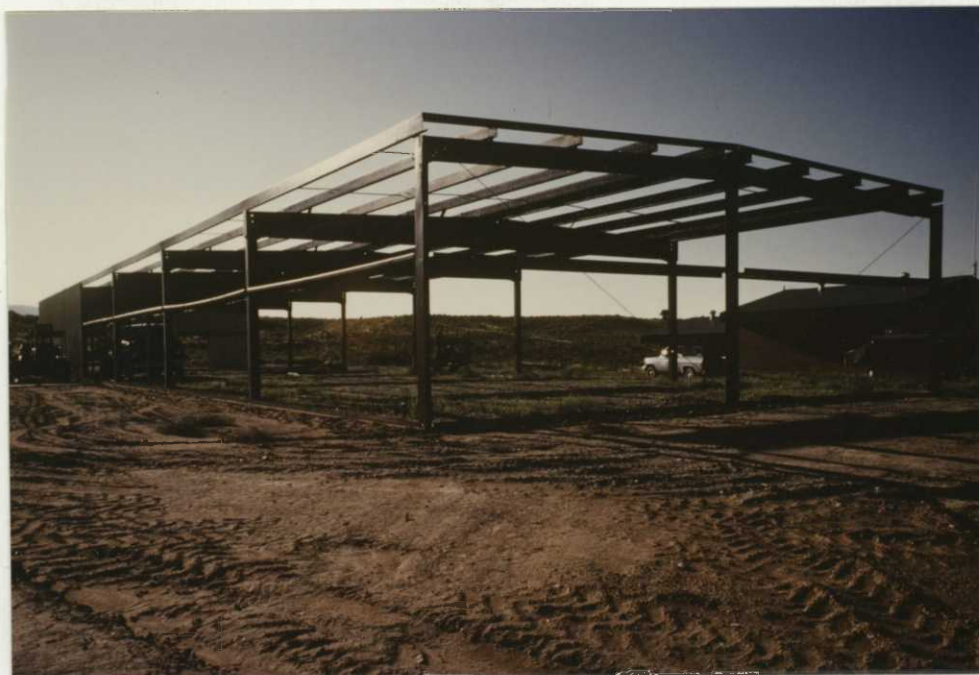
Photo 32. Work continued on the Butler building that was acquired surplus from Bear River MBR. 7/30/86, JC.
