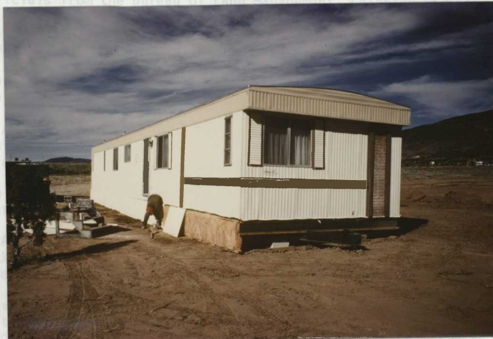
Photo 36. Joli Vollers puts skirting around the 14' X 70' mobile home we acquired surplus from the Bureau of Reclamation. It will be used to house temporary employees. 11/14/86-147, JC.
