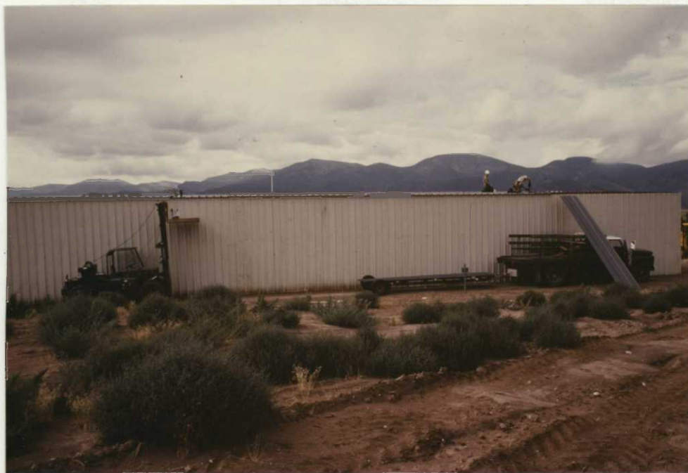
Photo 33. When we couldn't find anything else to do, we could always work on the Butler building. By the end of the year all we had left to do was put on the doors and windows. 8/86-80, JC
