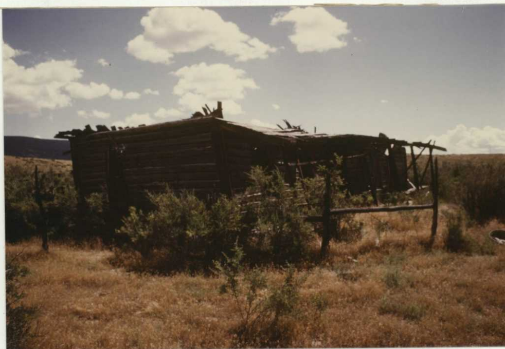
Photo 25. The Two-Bar ranch house is slowly deteriorating at one of the two historical sites on the refuge. 7/24/86-61, JC.
