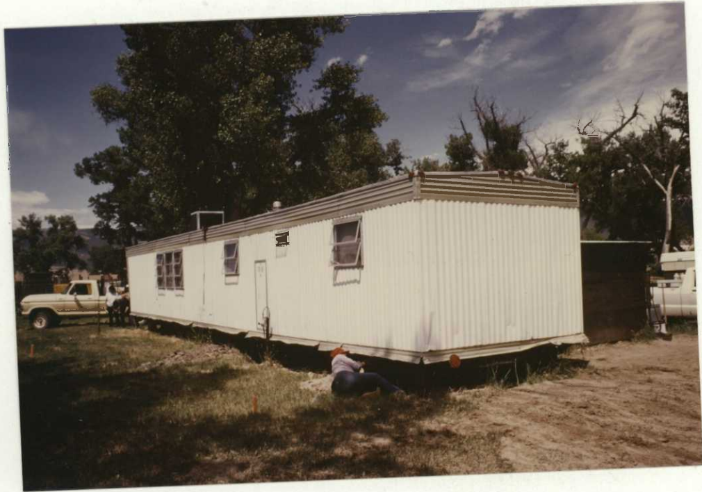
Photo 34. Preparing to move 10' X 55" mobile home for replacement with a 20' X 60' mobile home. 7/86-48, JC.
