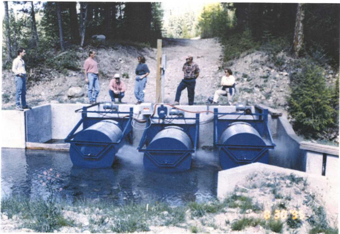
This fish friendly irrigation structure was installed on an irrigation canal diverting water from the Northfork of the Blackfoot River. The Northfork is a major bull trout spawning tributary. The structure uses stainless steel screens to prevent fish from swimming down the ditch. This $20K project was co-funded by Trout Unlimited, MDFWP and MT PFW. 9/95
