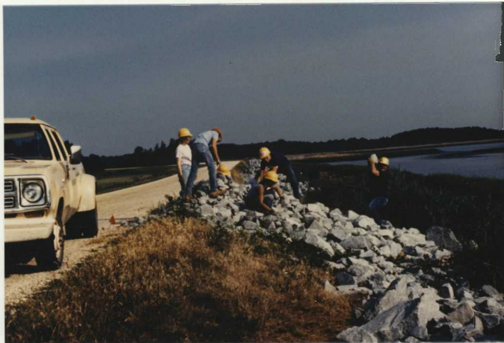
#32 Placement of 530 tons of rip-rap will make Sheariness Dike less prone to erosion caused by high tides and wave action.
