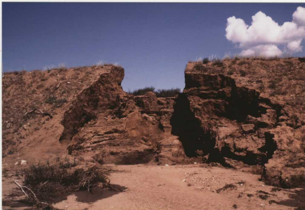
Water overfilled Lopez Tank and caused a major break in the dike. WAS
