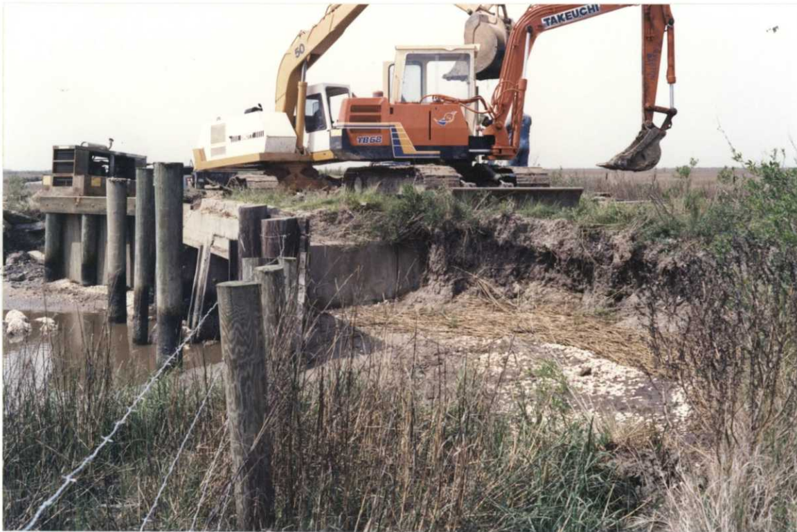
CONTRACTOR MOVING IN AT THE COON CREEK STRUCTURE SITE. THIS EXTENSIVE EROSION IS TYPICAL OF OTHER SITES.
