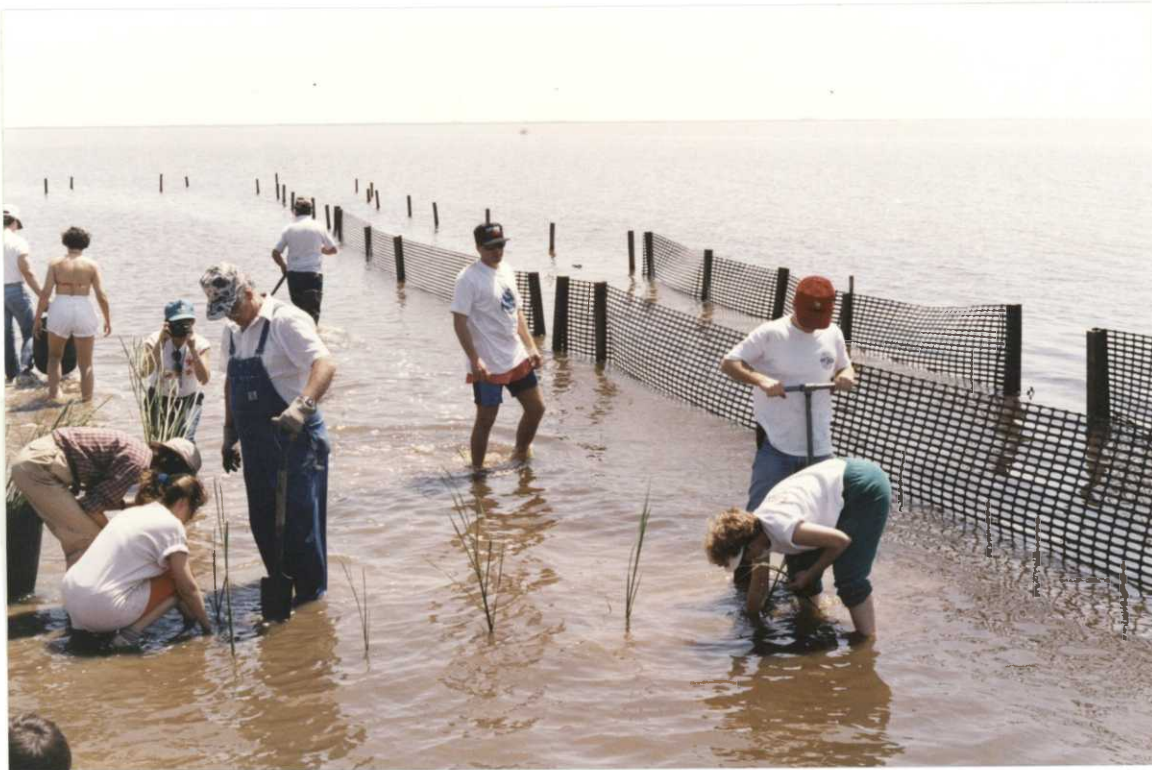
SMOOTH CORDGRASS BEING PLANTED BEHIND PARTIALLY COMPLETED WAVE ENERGY ABSORPTION FENCES ON THE SHORELINE OF EAST BAY
