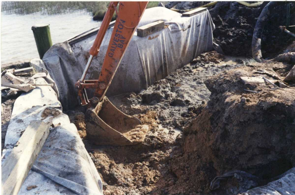
NEW BULKHEADS WERE COVERED WITH FILTER FABRIC. EXCAVATIONS WERE BACKFILLED WITH CEMENT REINFORCED SAND.
