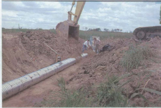
Goose Pen structure was just one of four replaced after 30 years of use. GDT
